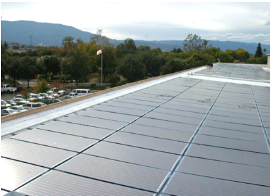
Rooftop solar array on Administration building
