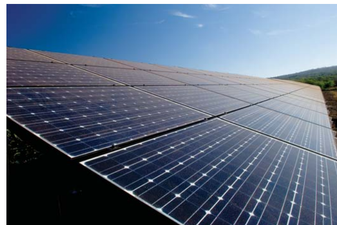
107 kW Waste Water reclamation Facility, Makena, 2009
