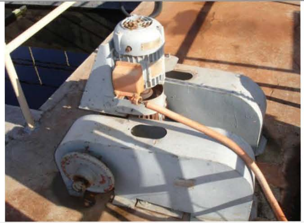
Existing Sludge Scraper Motor
