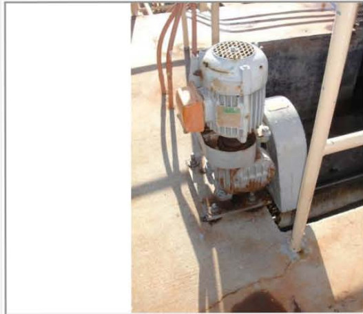
Existing Scum Collector Motor
