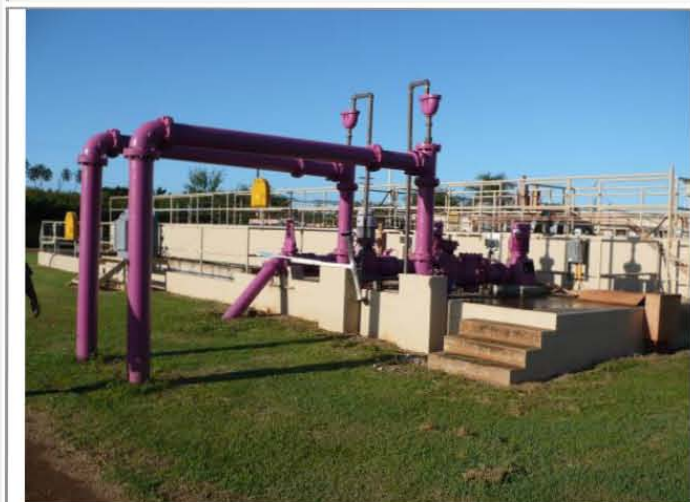
Existing Effluent Pumps and Motors
