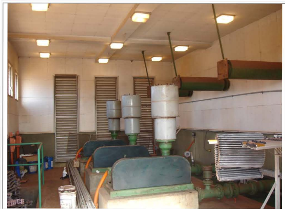
Existing 25 hp, constant speed, belt driven, 550 cfm blower units
