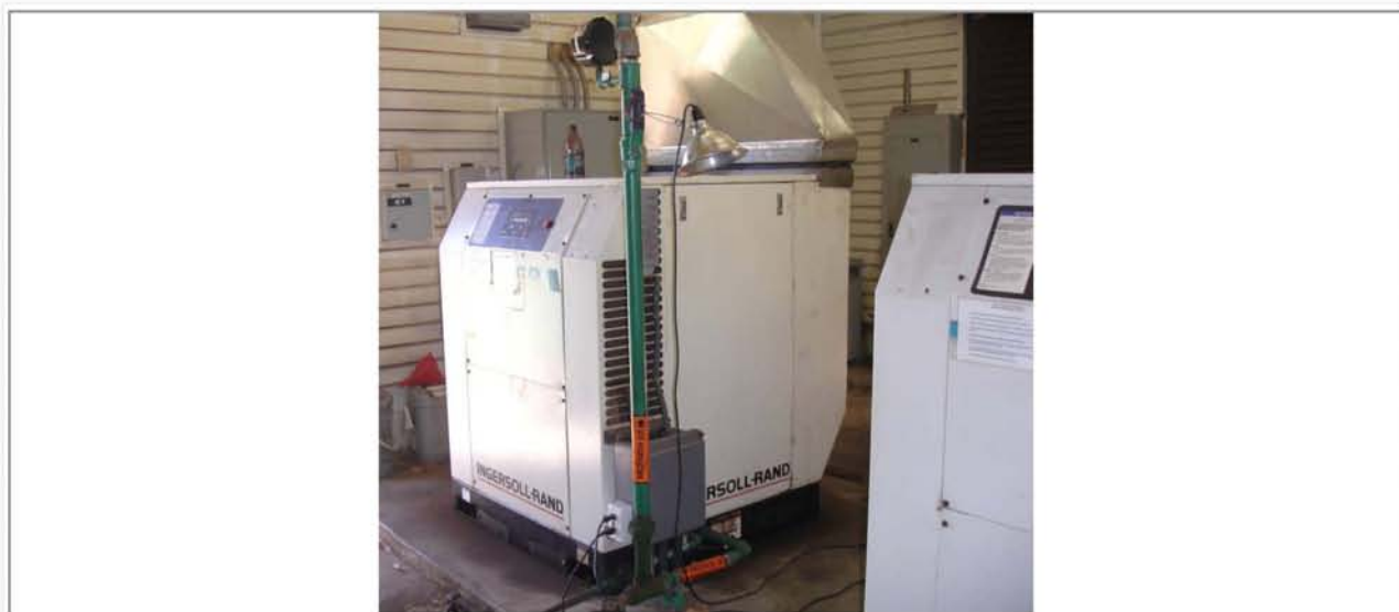
Sites Existing Compressors – Ingersoll Rand 40hp, Fixed Speed, Rotary Screws
