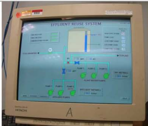
Existing Monitoring System for Effluent Reuse System
