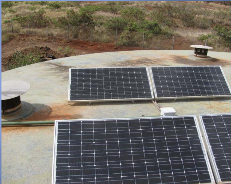
Solar panels that provide energy for SCADA equipment
