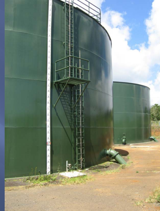
New steel reservoirs
