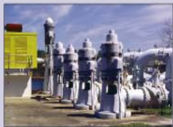
Public supply water intake, Bay County, Florida
