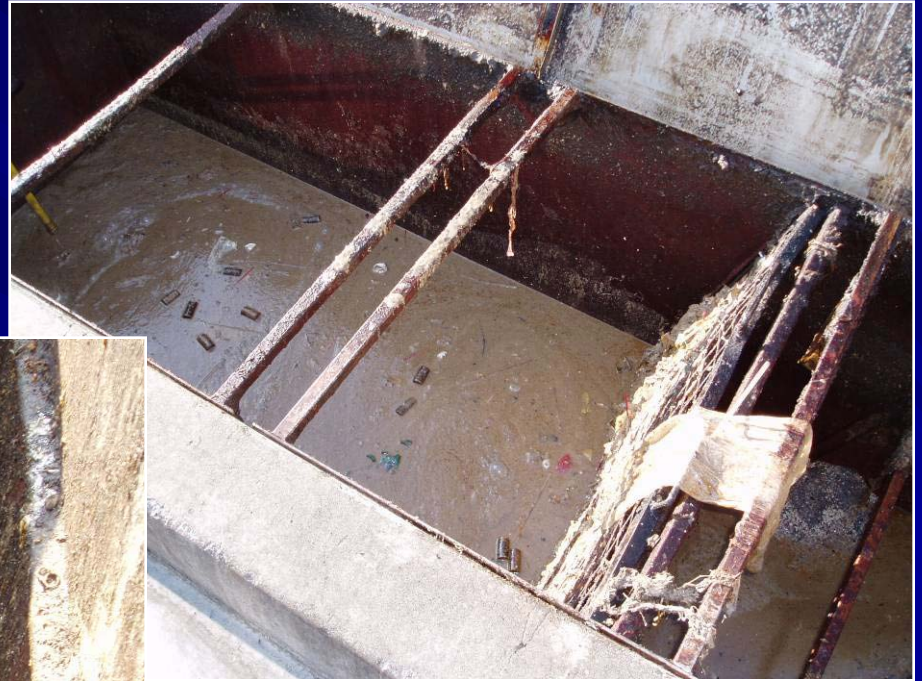
Grease trap waste
