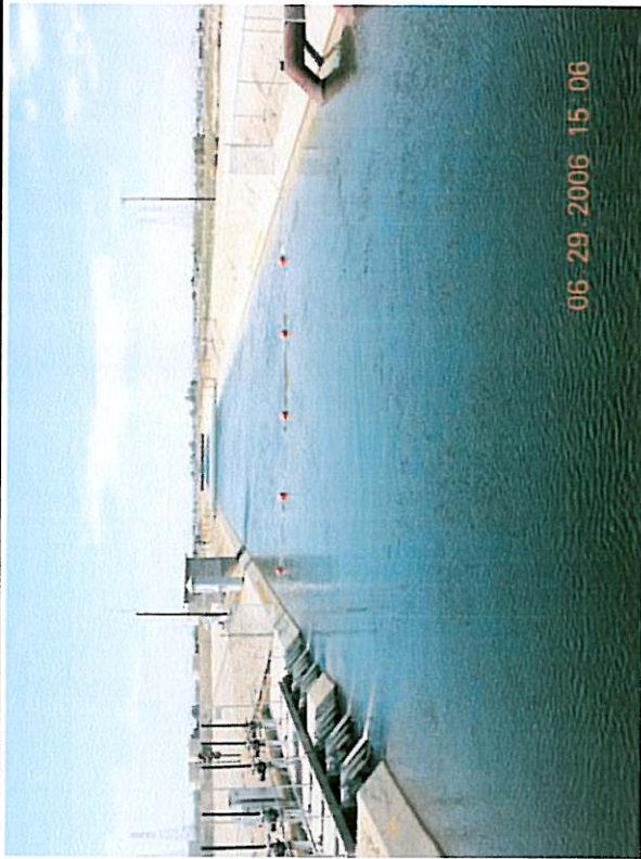
Friant-Kern Canal turn out into the Arvin-Edison Canal and siphon connection to the Cross Valley Canal.
