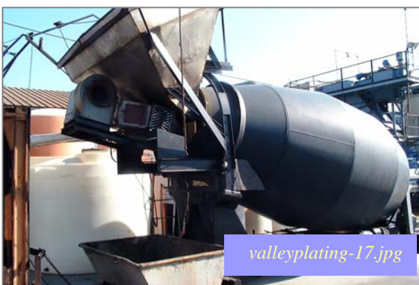
Photo #11: Rotating Sludge Dryer Taken By: Greg V. Arthur Date: 09/09/08
