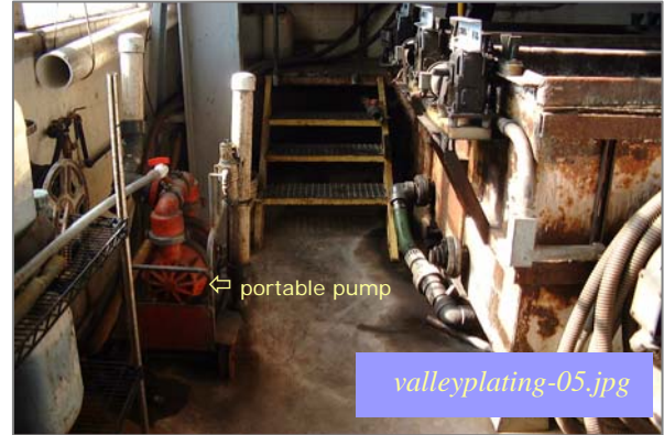
Photo #2: Line C - Portable Pump to Standpipe Taken By: Greg V. Arthur Date: 09/09/08
