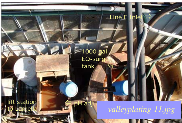
Photo #9: IWTP - Metals Precipitation Taken By: Greg V. Arthur Date: 09/09/08
