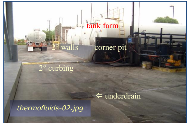
Photo #2: Truck Receiving Loading Rack Taken By: Greg V. Arthur Date: 08/13/09
