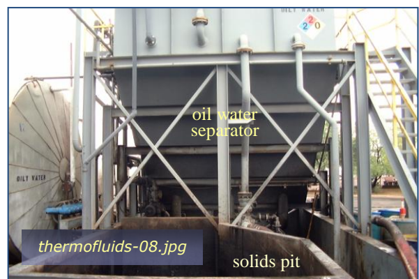
Photo #6: Oily Wastewater Treatment - O/W Sep Taken By: Greg V. Arthur Date: 08/13/09
