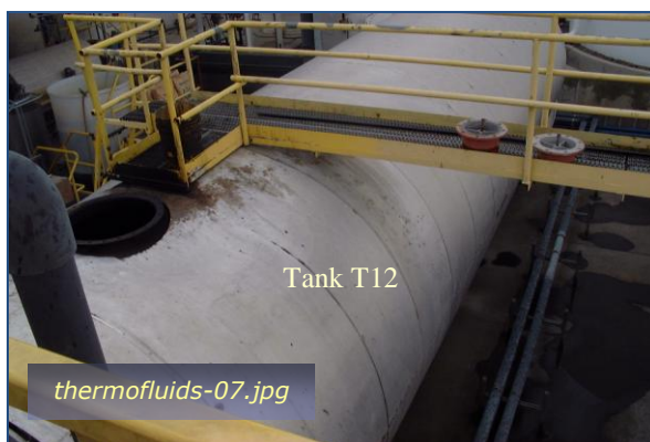
Photo #5: Oily Wastewater Treat - De-emulsifier Taken By: Greg V. Arthur Date: 08/13/09
