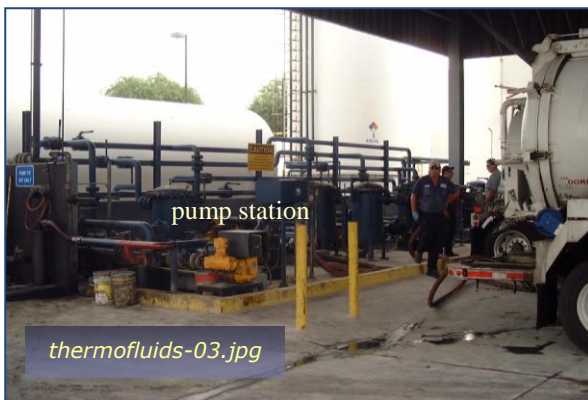
Photo #3: Truck Receiving Pump Station Taken By: Greg V. Arthur Date: 08/13/09
