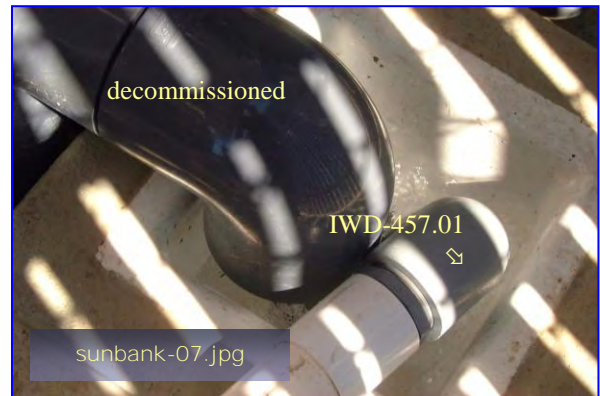
Photo #8: Bldg 1730 - Discharge (IWD-457.01) Taken By: Greg V. Arthur Date: 08/10/11
