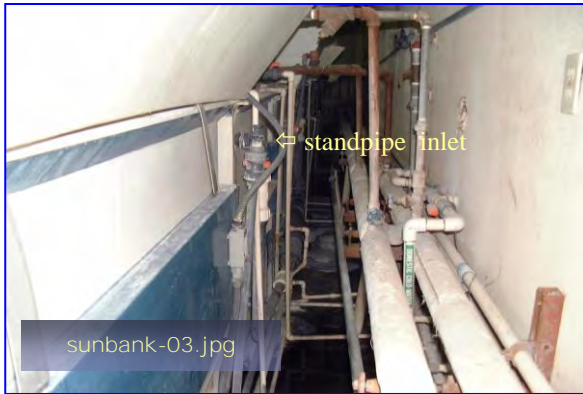
Photo #3: Bldg 1730 – Plating Spents Standpipe Taken By: Greg V. Arthur Date: 08/10/11
