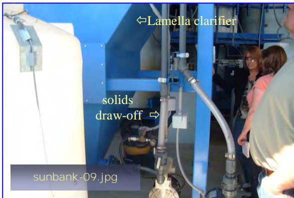
Photo #7: Bldg 1730 - IWTP Lamella clarifier Taken By: Greg V. Arthur Date: 08/10/11
