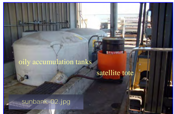
Photo #2: Bldg 1740 - Oily Accumulation Tanks Taken By: Greg V. Arthur Date: 08/10/11
