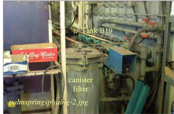
Photo: Ni-Plating Tank B19 Circulation Filter Taken By: Greg V. Arthur Date: 10/08/07
