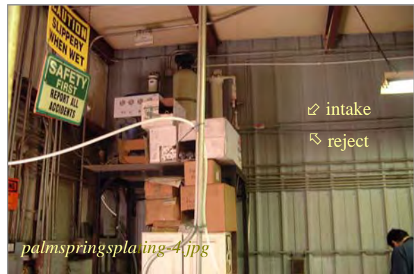
Photo: RO Preconditioning Unit for City Water Taken By: Greg V. Arthur Date: 010/08/07
