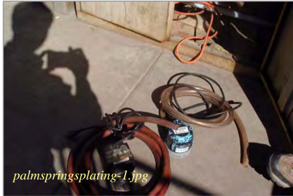
Photo: Solution Transfer Pumps and Hoses Taken By: Greg V. Arthur Date: 10/08/07
