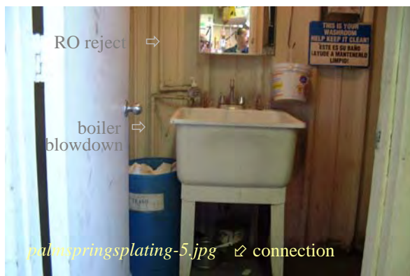
Photo: Work Sink and Connection to the Sewer Taken By: Greg V. Arthur Date: 10/08/07
