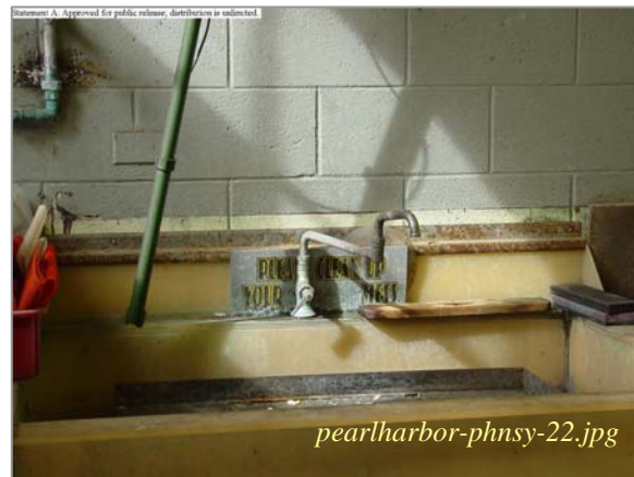
Photos: Bldg 67 - Brushplating Table and Sink Discharge to the 5,000 gal Holding Tank Taken By: Christie Chun, PHNSY Date: 04/12/06
