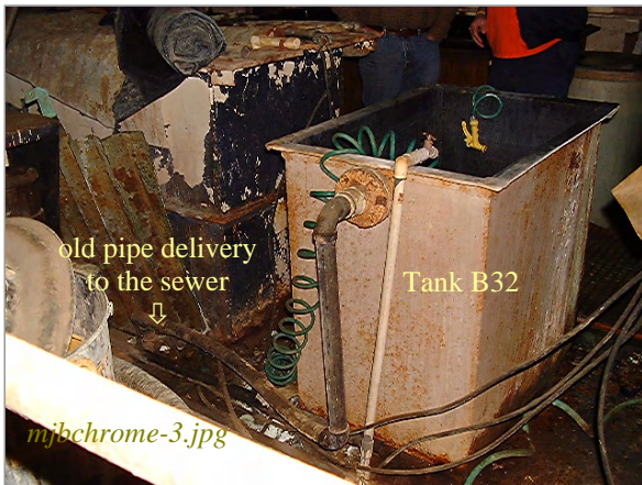
Photo: Hard-piping from Rinse Tank B32 to sewer Taken By: Greg V. Arthur Date: 04/17/07
