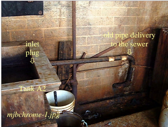
Photo: Hard-piping from Rinse Tank A2 to sewer Taken By: Greg V. Arthur Date: 04/17/07
