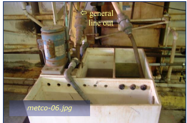
Photo #4: Old-Site Weir Box D to IWTP Taken By: Greg V. Arthur Date: 09/23/09
