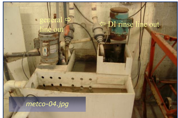
Photo #2: Old-Site Weir Box B to IWTP Taken By: Greg V. Arthur Date: 09/23/09
