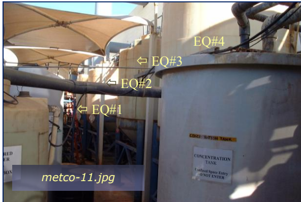
Photo #7: IWTP Equalization Tanks Taken By: Greg V. Arthur Date: 09/23/09
