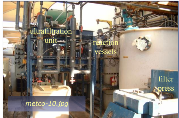
Photo #8: IWTP Unit Processes Taken By: Greg V. Arthur Date: 09/23/09
