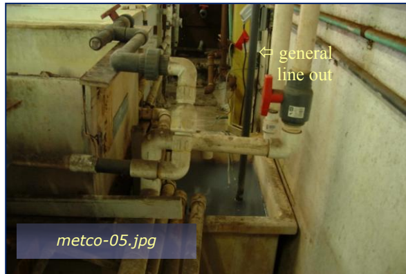
Photo #3: Old-Site Weir Box C to IWTP Taken By: Greg V. Arthur Date: 09/23/09
