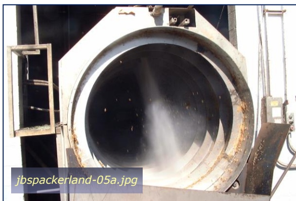
Photo #5: IWTP Rotoscreen Taken By: Greg V. Arthur Date: 08/14/09
