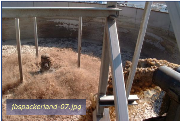
Photo #7: IWTP Aerated Surge Tank Taken By: Greg V. Arthur Date: 08/14/09
