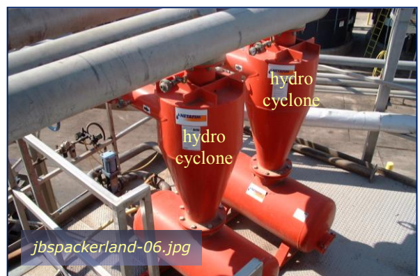
Photo #6: IWTP Hydrocyclones Taken By: Greg V. Arthur Date: 08/14/09
