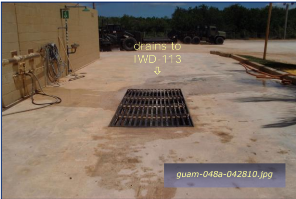
Photo #4-31: Bldg 563 Outdoor Washrack Taken By: Greg V. Arthur Date: 04/28/10
