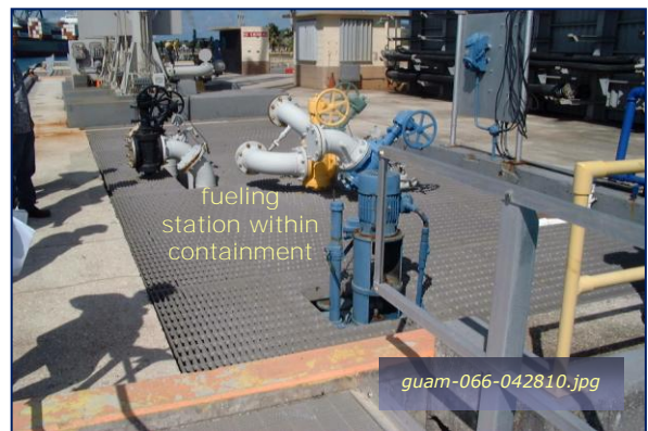
Photo #4-16: FISC Fueling Pier – Containment Drain Taken By: Greg V. Arthur Date: 04/28/10
