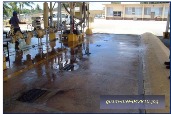
Photo #4-14: FISC Fuel Farm – Bottom Fill Drains Taken By: Greg V. Arthur Date: 04/28/10
