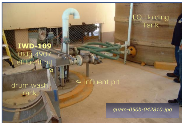
Photo #4-27: Bldg 4907 Demin Plant - Discharge Taken By: Greg V. Arthur Date: 04/28/10
