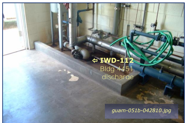
Photo #4-30: Bldg 4451 Steam Plant - Boiler Line 2 Taken By: Greg V. Arthur Date: 04/28/10
