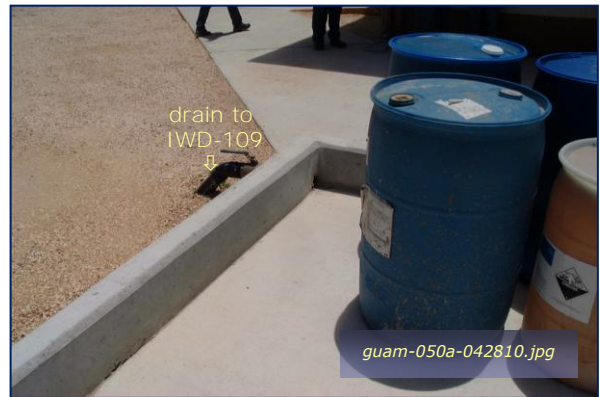
Photo #4-26: Bldg 4907 Demin Plant - Rack Drain Taken By: Greg V. Arthur Date: 04/28/10
