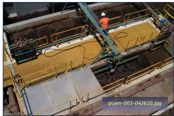
Photo #3-2: Activated Sludge – Solids Contact Taken By: Greg V. Arthur Date: 04/26/10
