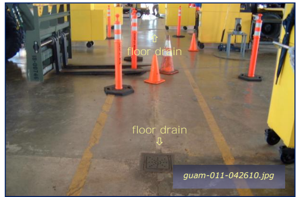
Photo #4-20: Bldg 364 Motor Pool – Floor Drains Taken By: Greg V. Arthur Date: 04/26/10
