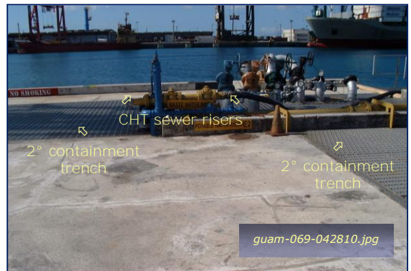
Photo #3-10: Echo Fueling Pier CHT Sewer Riser Taken By: Greg V. Arthur Date: 04/28/10
