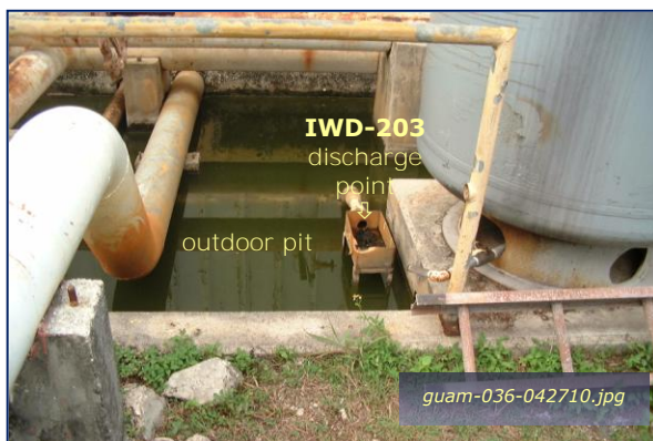
Photo #5-5: Bldg 2078 Compressor Plant Taken By: Greg V. Arthur Date: 04/27/10
