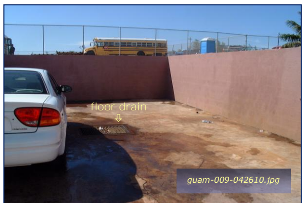
Photo #4-22: Bldg 372 Outdoor Washrack Taken By: Greg V. Arthur Date: 04/26/10
