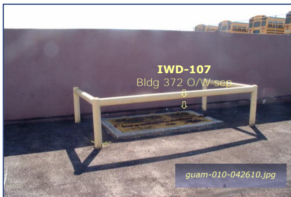
Photo #4-21: Bldg 372 Outdoor Washrack - O/W Sep Taken By: Greg V. Arthur Date: 04/26/10
