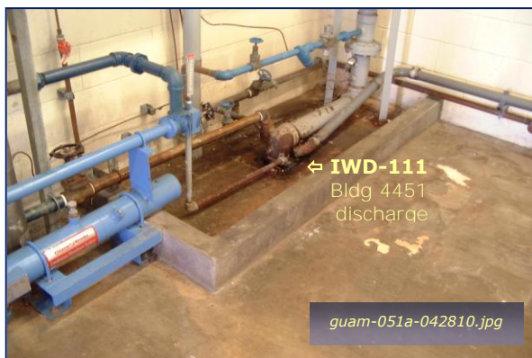
Photo #4-29: Bldg 4451 Steam Plant - Boiler Line 1 Taken By: Greg V. Arthur Date: 04/28/10
