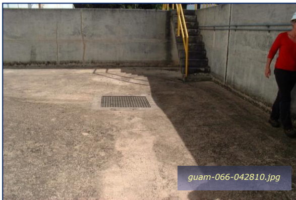
Photo #4-15: FISC Fuel Farm – Tank Berm Drain Taken By: Greg V. Arthur Date: 04/28/10
