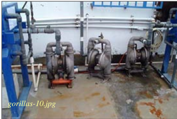
gorillas-10.jpg Photo #5: Portable pumps on standby Taken By: Greg V. Arthur Date: 09/11/08
