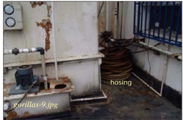
gorillas-9.jpg Photo #6: Flexible hosing for portable pumps Taken By: Greg V. Arthur Date: 09/11/08
