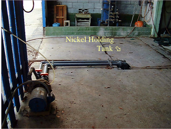
Photo: Nickel-Bearing Sump and Pump Taken By: Greg V. Arthur Date: 09/07/06
