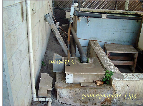
Photo: Sample Box and Sewer Connection Taken By: Greg V. Arthur Date: 09/07/06
