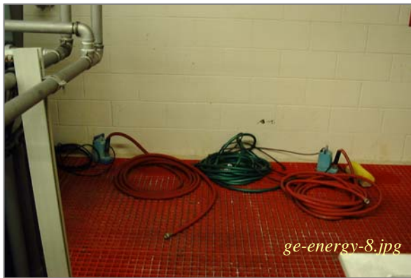
Photo: Anodizing Room - Portable Pumps / Hoses Taken By: Greg V. Arthur Date: 11/27/07
