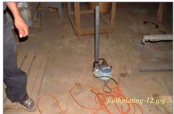
Photo: Portable pump and riser for connection Taken By: Greg V. Arthur Date: 010/09/07
