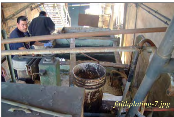
Photo: Industrial wastewater treatment unit Taken By: Greg V. Arthur Date: 10/09/07
