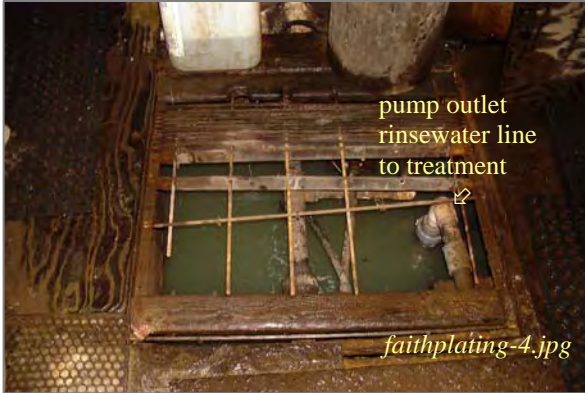
Photo: Underfloor drainage sump to treatment Taken By: Greg V. Arthur Date: 10/09/07
