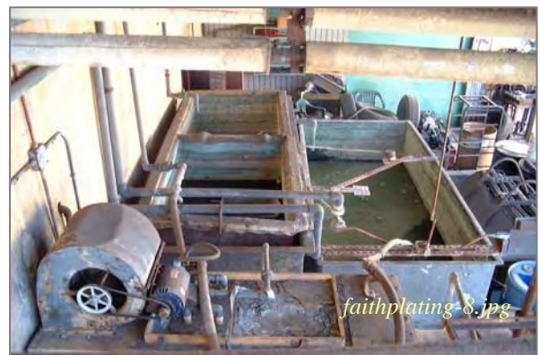
Photo: Dedicated batch treatment tanks Taken By: Greg V. Arthur Date: 10/09/07
