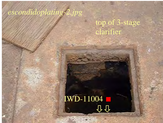
Photo: Final Clarifier Taken By: Greg V. Arthur Date: 05/02/07
