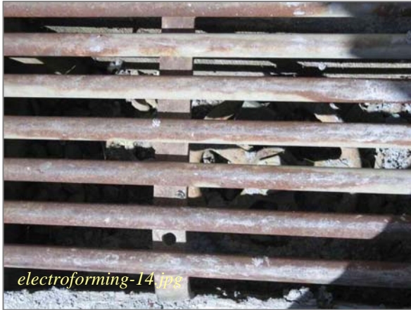
Photo: Sewer Connection - Sealed and Locked Taken By: Anna Yen Date: 08/28/07
