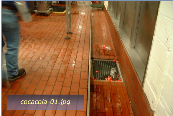
Photo #1: Floor Drains on Shop Floor Taken By: Greg V. Arthur Date: 09/24/09
