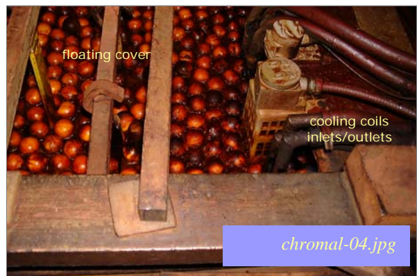
Photo #6: Chrome Tank Source Controls Taken By: Greg V. Arthur Date: 09/10/08
