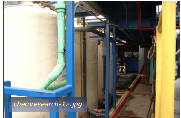
Photo #8: Equalization Tanks 1 through 3 Taken By: Greg V. Arthur Date: 08/13/09
