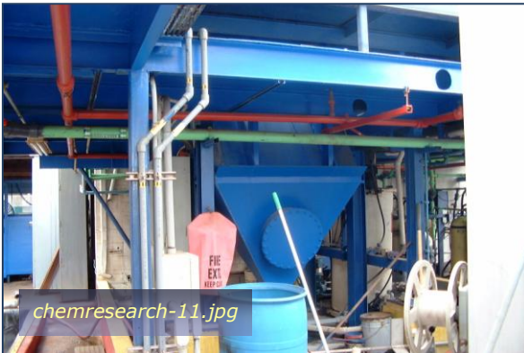
Photo #9: IWTP Lamella Clarifier Taken By: Greg V. Arthur Date: 08/13/09
