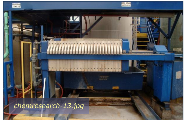
Photo #10: IWTP Filter Press Taken By: Greg V. Arthur Date: 08/13/09
