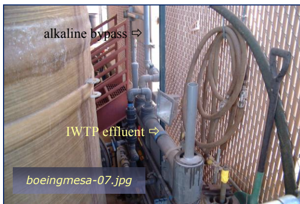
Photo #3: IWTP Effluent Line to In-Plant Sewer Taken By: Greg V. Arthur Date: 09/25/09
