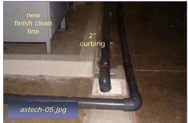
Photo #6: Floor Drain for New Finish Clean Line Taken By: Greg V. Arthur Date: 09/12/08
