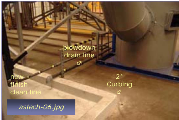
Photo #5: Fume Scrubber Blowdown Taken By: Greg V. Arthur Date: 09/12/08
