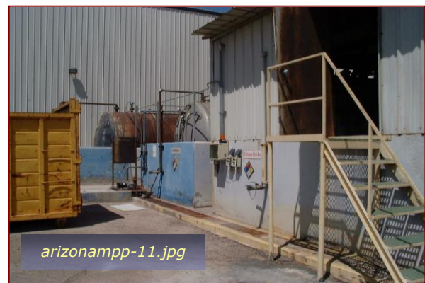
Photo #10: Outside Chemical Storage Area Photo Taken By: Greg V. Arthur Date: 08/12/09
