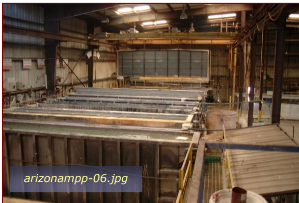
Photo #1: Metal Finishing Tanks Taken By: Greg V. Arthur Date: 08/12/09
