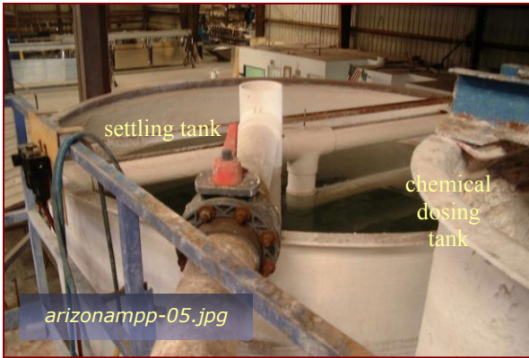
Photo #5: IWTP Settling Tank and Reaction Tank Taken By: Greg V. Arthur Date: 08/12/09
