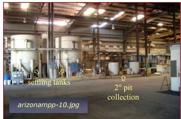
Photo #4: IWTP – reaction/settling/2°pit Taken By: Greg V. Arthur Date: 08/12/09
