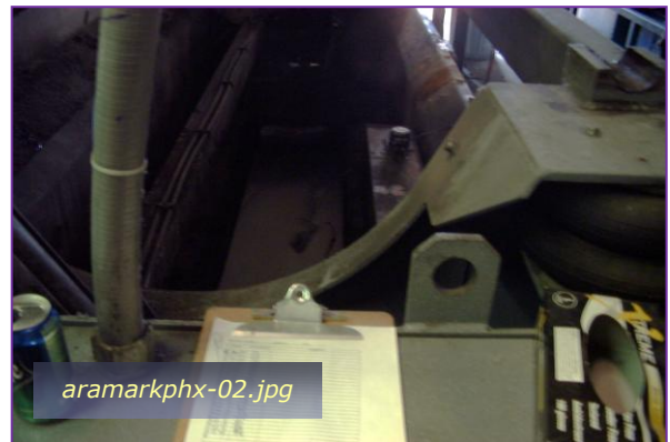
Photo #2: Drainage Trench Behind Washer Taken By: Greg V. Arthur Date: 09/23/09
