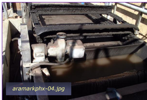
Photo #3: Induced Air Flotation Unit Taken By: Greg V. Arthur Date: 09/23/09
