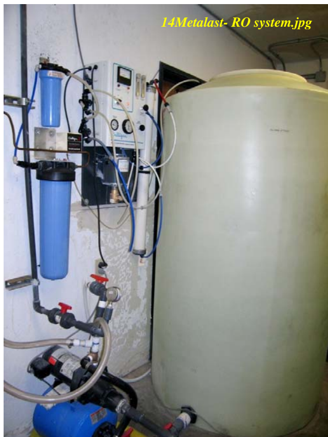
Photo 6 RO/DI system, with storage tank Taken by Anna Yen on May 21, 2008
