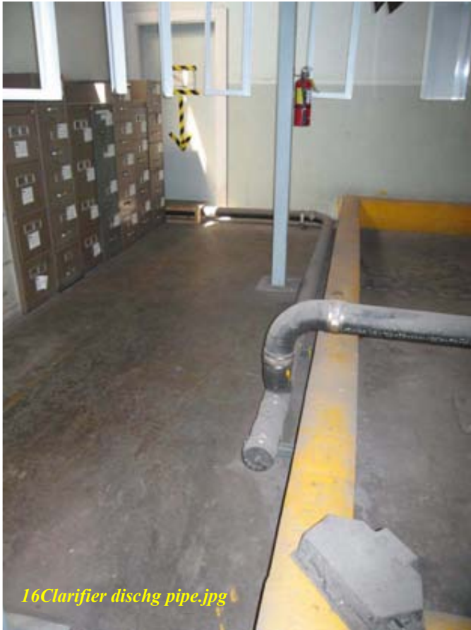
Photo 4 Discharge pipe from clarifier to outside building Taken by Anna Yen on August 24, 2010
