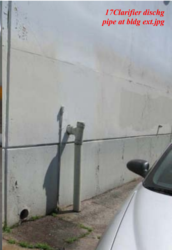
Photo 5 Clarifier discharge pipe outside of building - leading down to local sewer system Taken by Anna Yen on August 24, 2010
