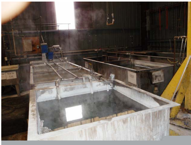
IVD aqueous degreaser tank and rinse tank
