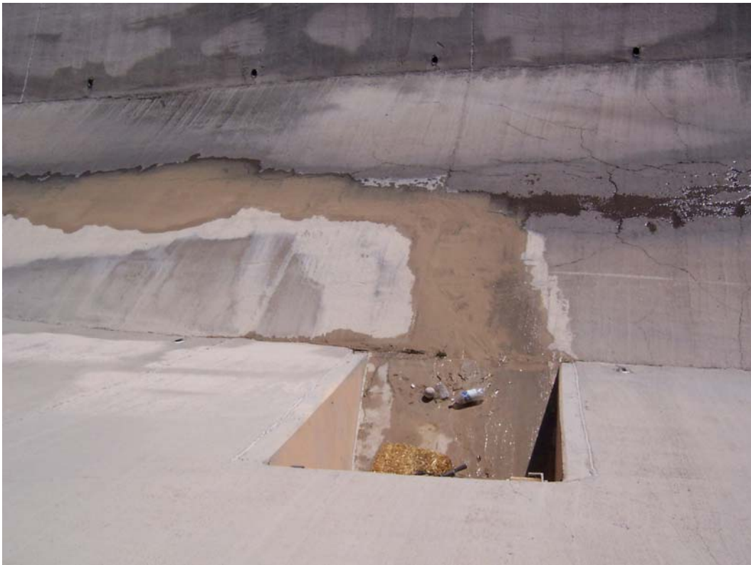
Photo 1. Water and sediment from the construction site entering the wash.
