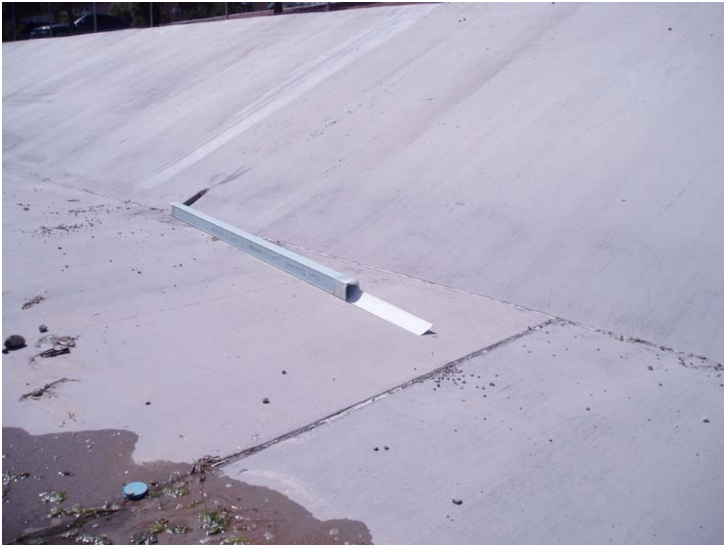
Photo 21. Empty box dumped in channel.
