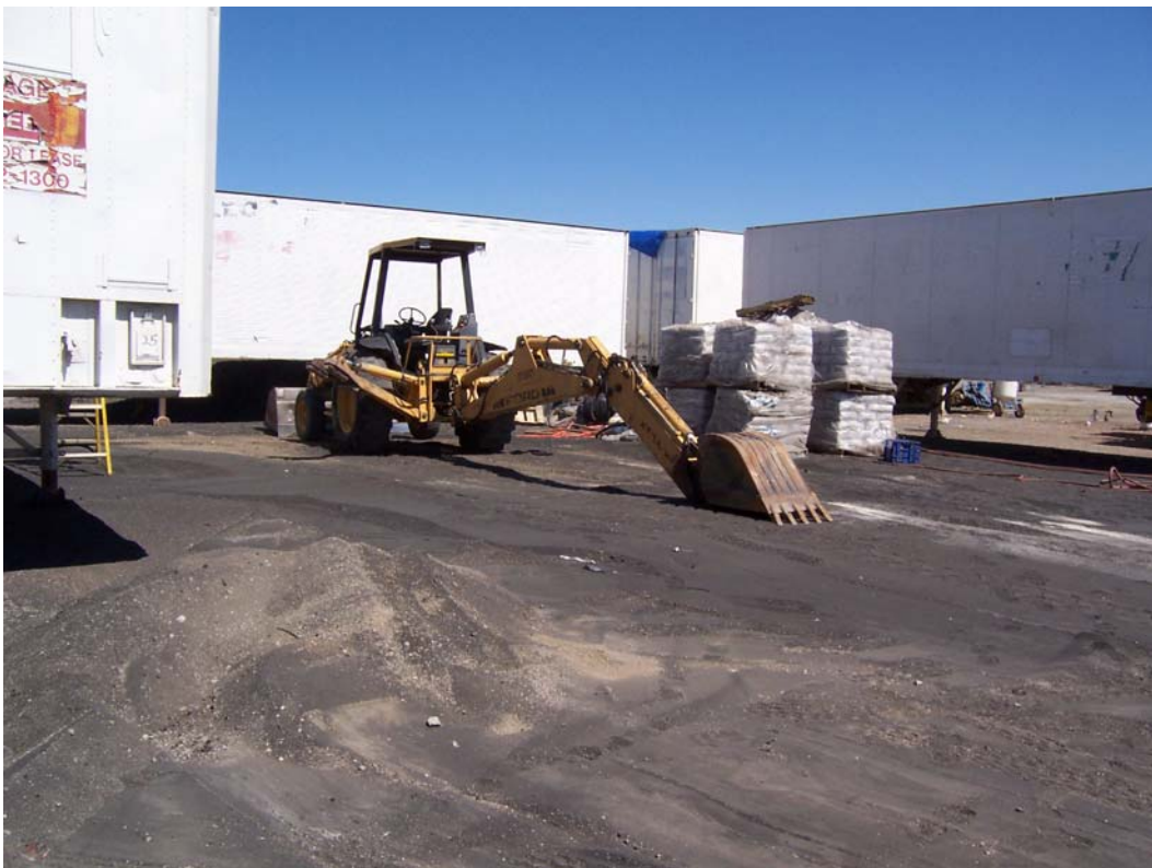
Photo 1. Open air sand blasting activity at the site. Dark material around the backhoe being sand blasted is spent sand blast grit. White bags on pallets at photo right are additional unused grit. No containment was provided around the area.
