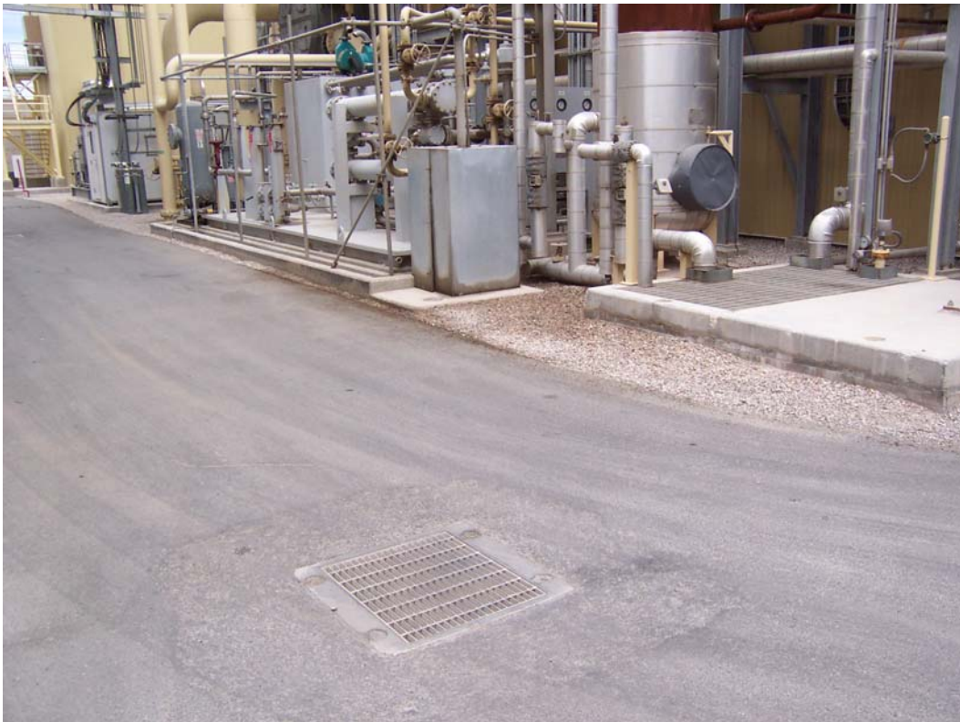
Photo 3. The inspector noted the presence of oil stains (center photo) on the rock landscaping and an electrical cabinet next to turbine number one.
