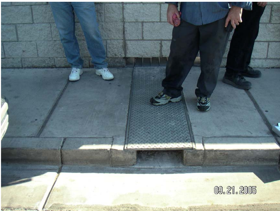
Photo 8. Dried milk solids entered street gutter from facility drain.
