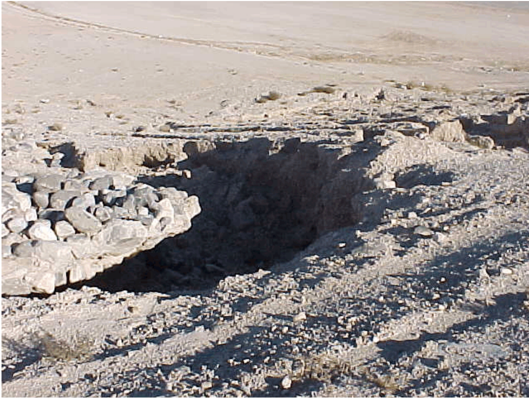
Photo 9. Erosion on west wall of detention basin.
