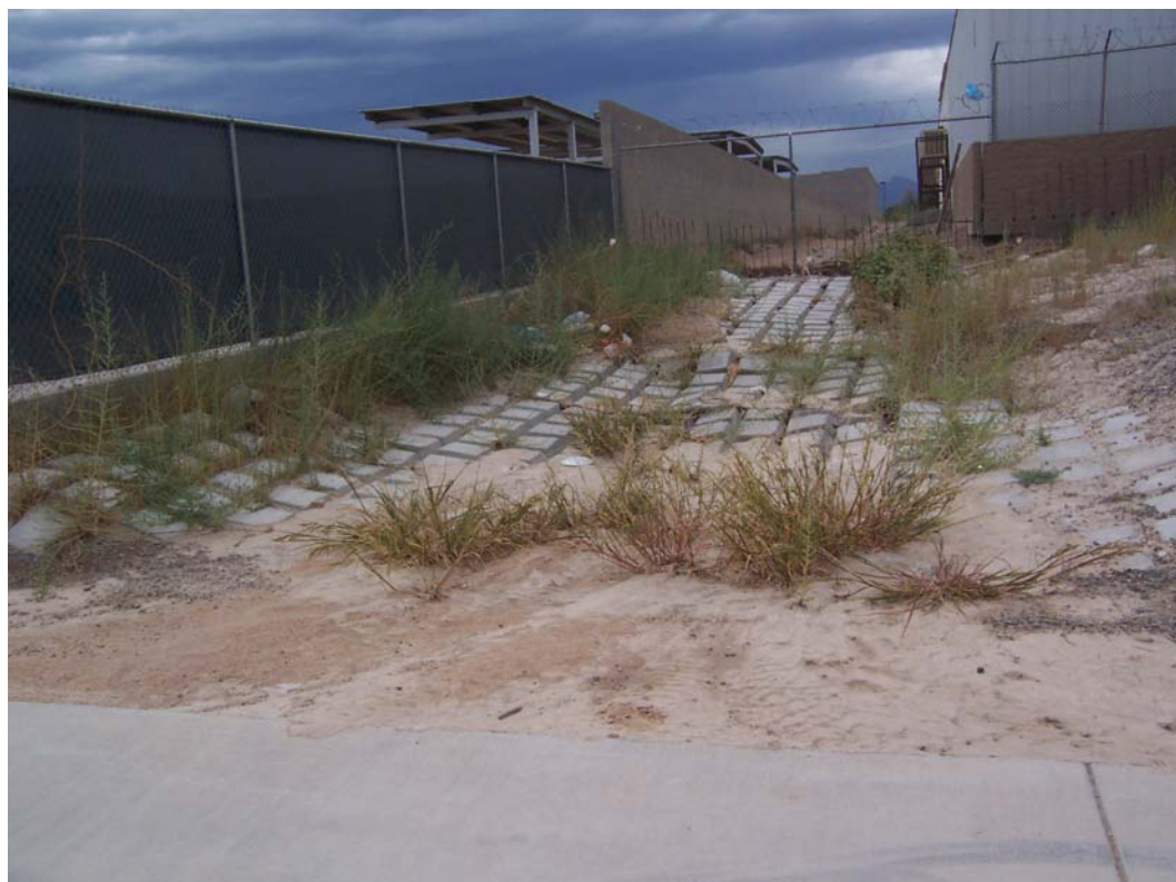
Photo 4. Riprap channel between commercial properties. Note lower end of channel appears to be clogged with sediment.
