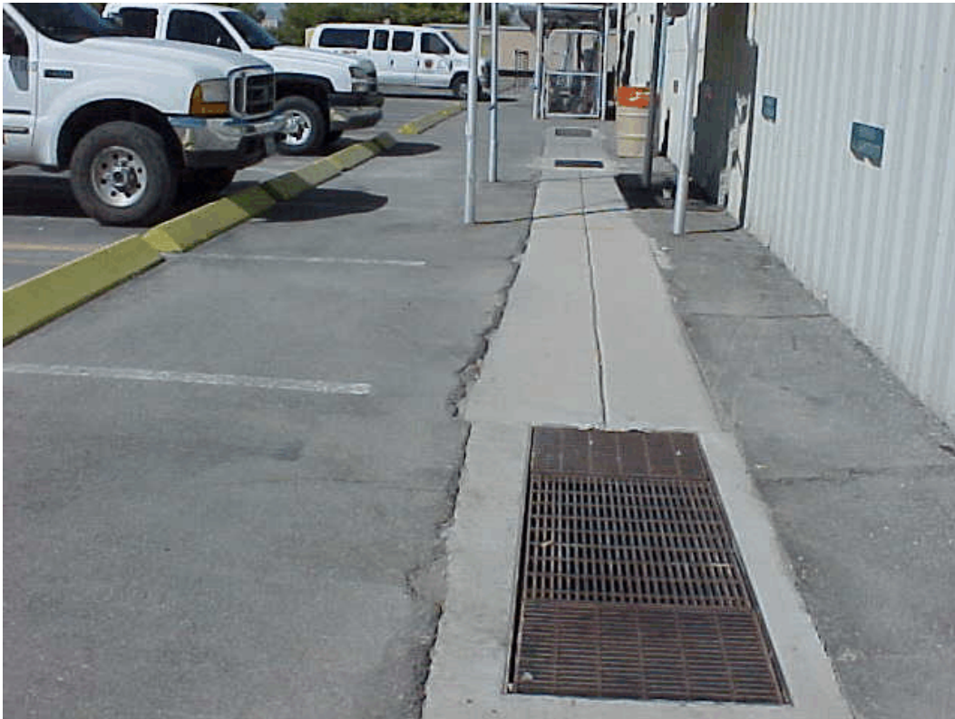
Photo 1. Fleet (primary) facility: Unprotected storm water inlets at north edge of parking area.
