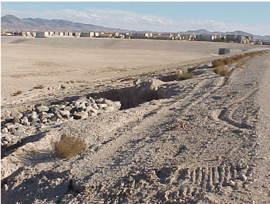
Photo 8. Erosion on west wall of detention basin.
