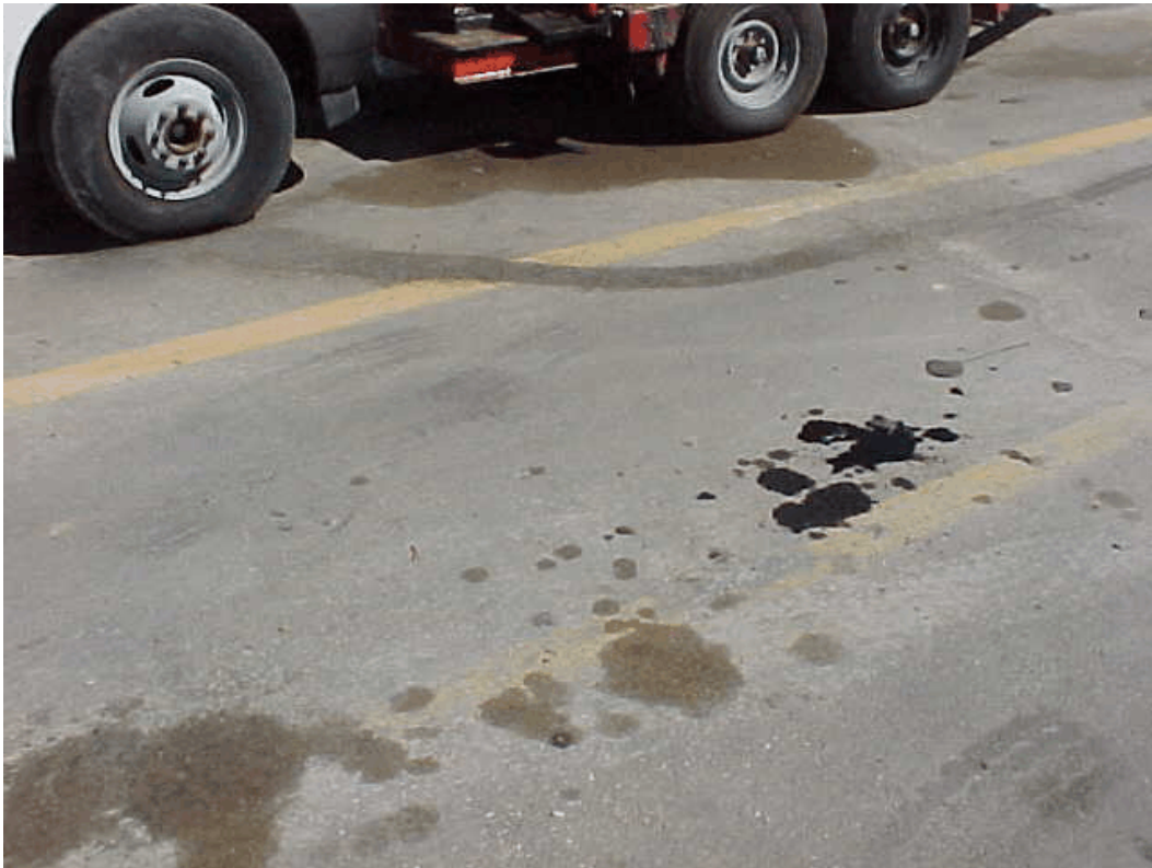
Photo 9. Fleet (primary) facility: Truck parking area with spills/leakage staining on pavement.
