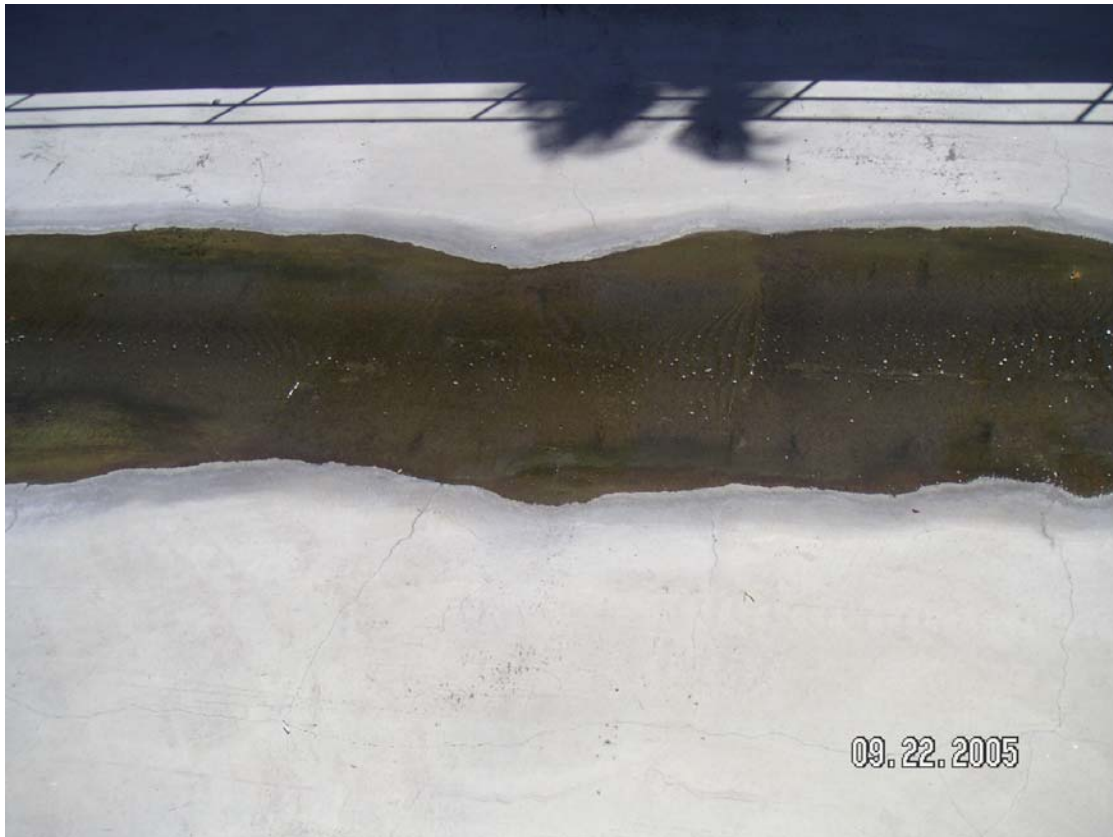
Photo 11. Meadows Detention Basin - flow in influent channel.
