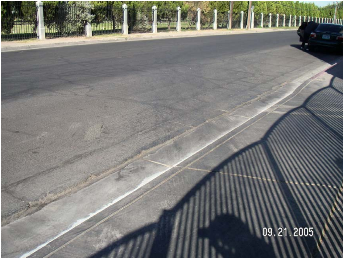
Photo 7. Dried milk solids in street gutter outside facility.
