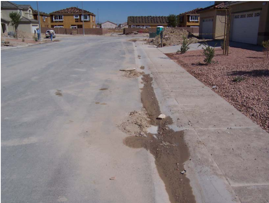
Photo 5. Sediment in the street. Moisture indicates street was washed earlier in the day. Note sand bag, center rear of photo, pulled back from the curb.
