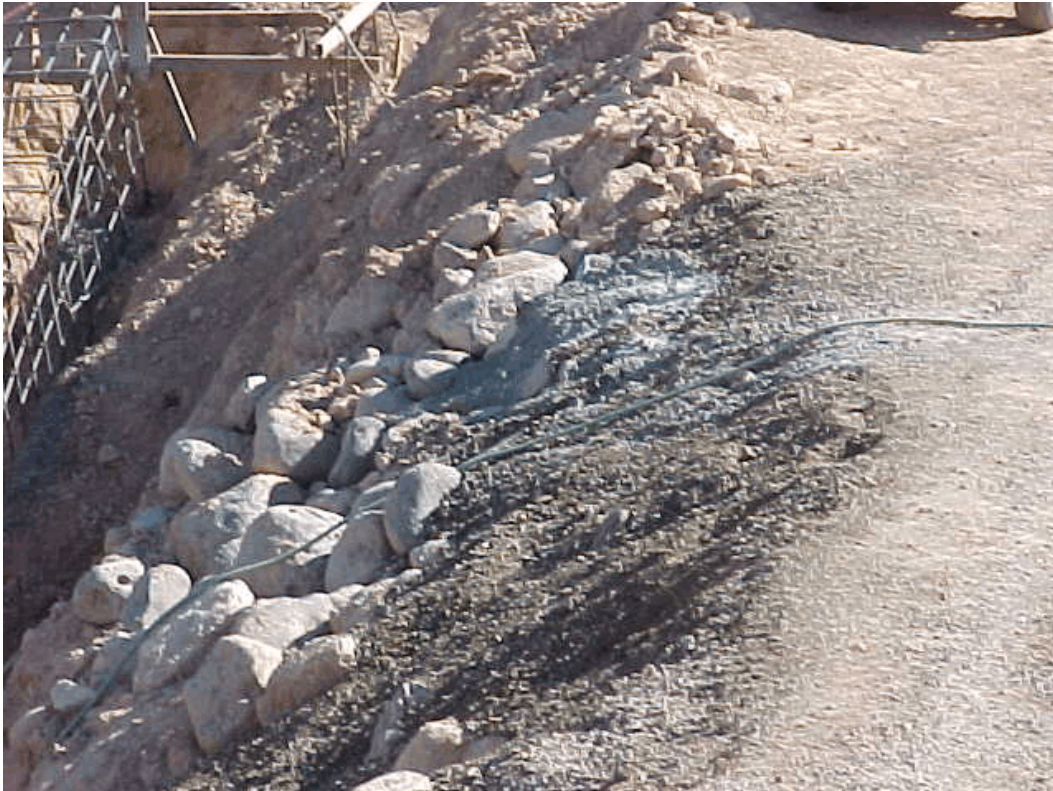
Photo 3. Closeup view of concrete washout on downstream face of earthen dam. A sump is located at the toe of the dam face (photo left).
