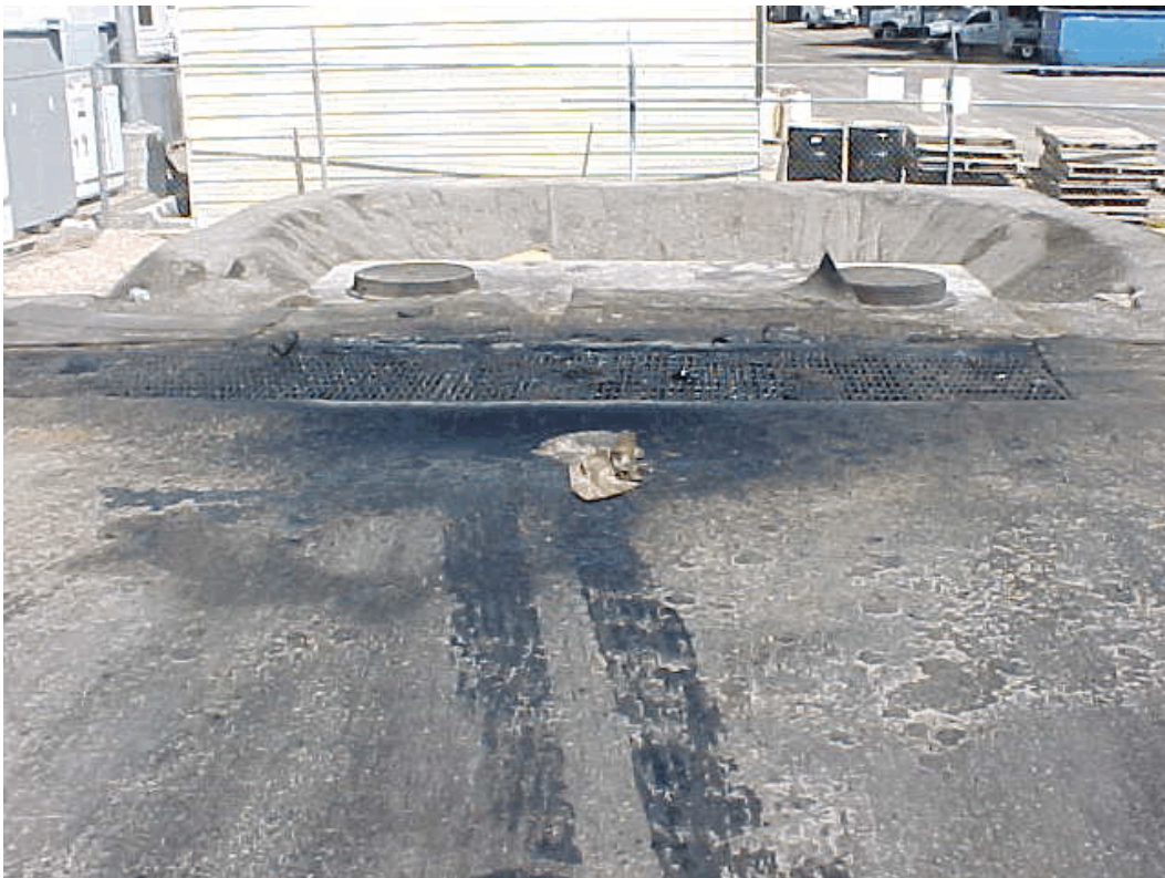
Photo 16. Fleet (secondary) facility: Abandoned asphalt washout area.
