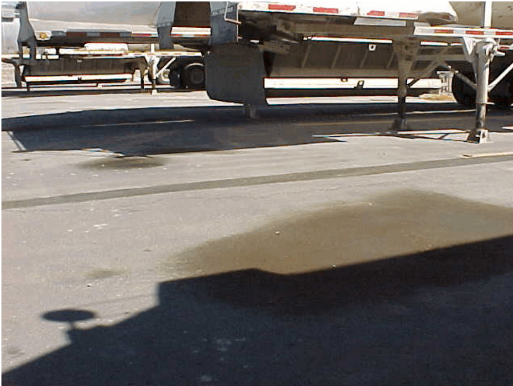
Photo 13. Fleet (secondary) facility: Truck and paving equipment parking area with spills/leakage staining on pavement.
