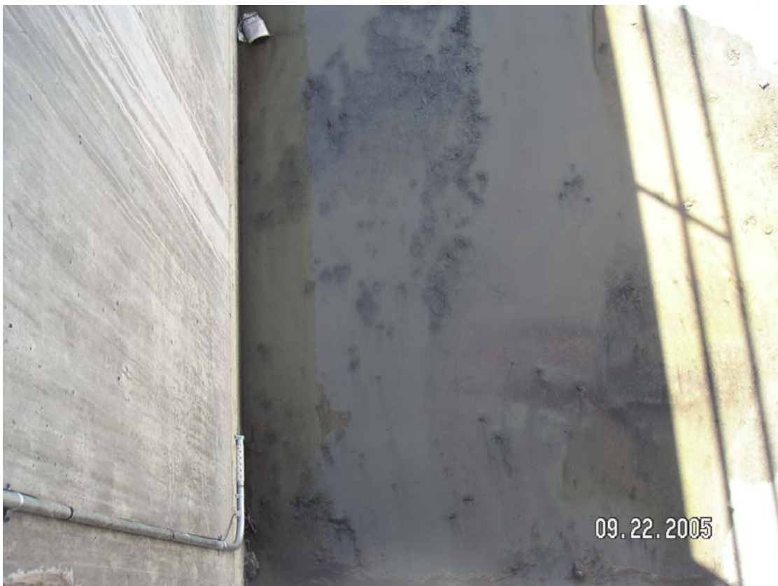
Photo 14. Meadows Detention Basin - effluent sample probe.
