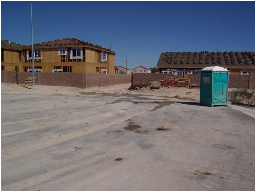
Photo 4. Portable toilet placed where spillage would go directly to storm inlet. Storm inlet is left center photo, at the end of the sidewalk to the cul-de-sac.
