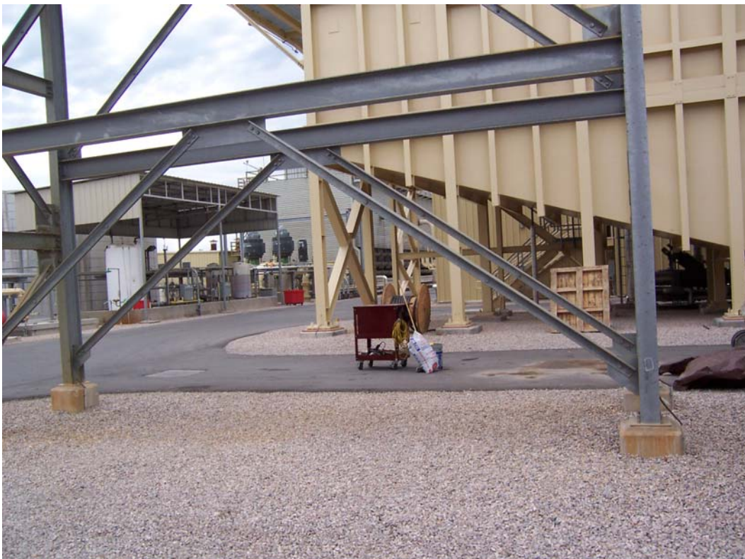
Photo 4. The inspector did note some oil spills on the pavement where adsorbent had been applied. He advised the facility to sweep up the adsorbent.
