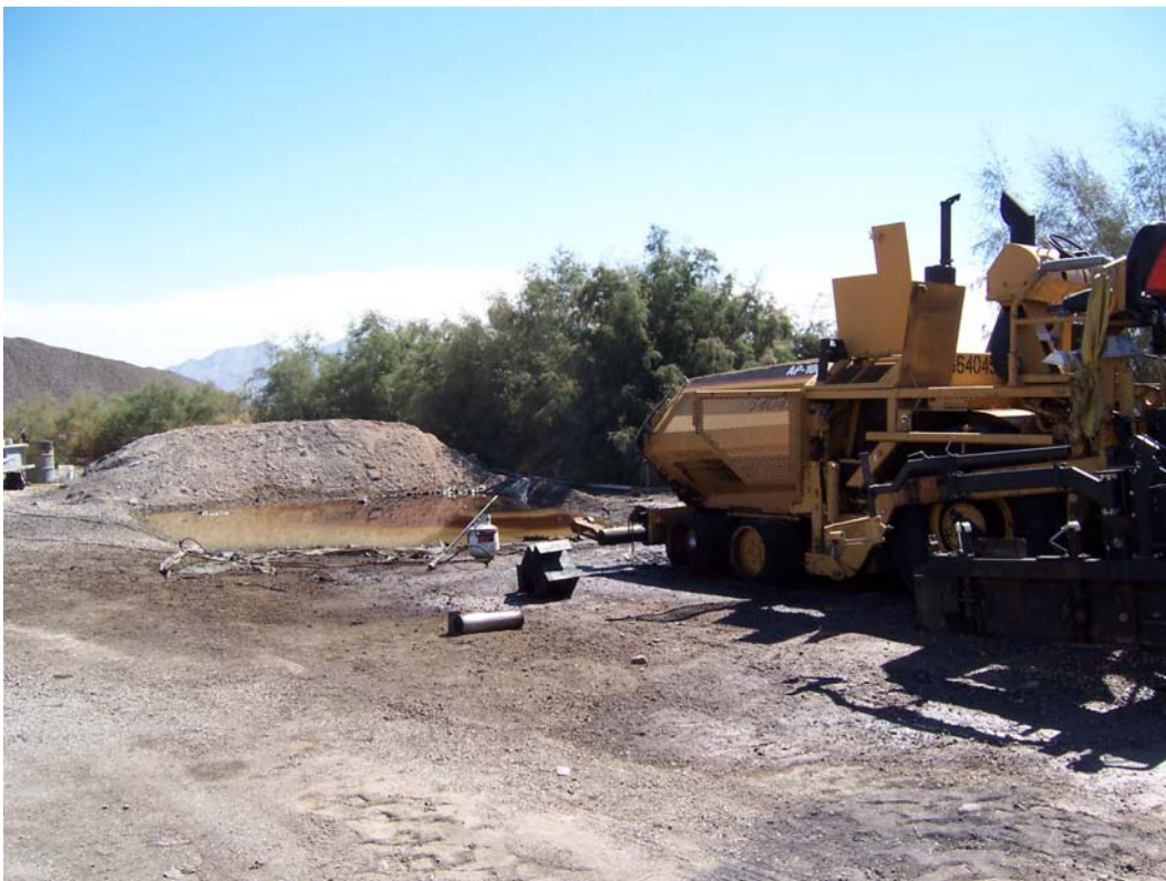
Photo 4. Paving machine being cleaned with wash water discharged to the pit shown in Photo 3. Note oil stains on the ground in front of and around the machine.
