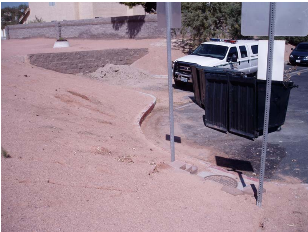
Photo 8. Parks and Recreation Department dirt storage. Trackout visible to inlet, which flows to outfall in Photo 7.
