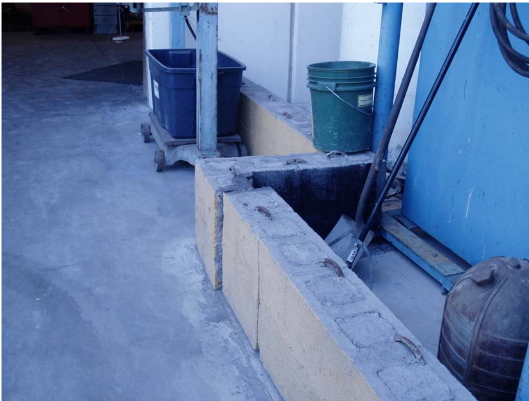
Photo 1. Crack in secondary containment.
