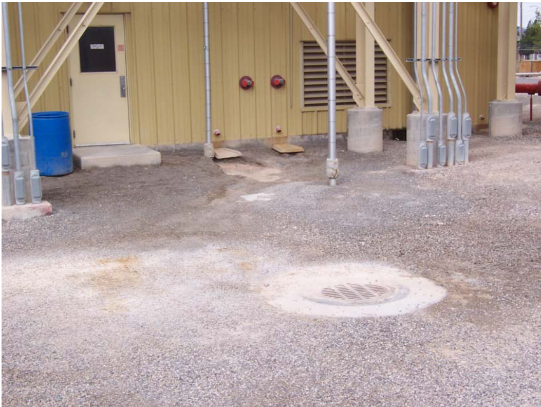
Photo 1. Inspector did not note evidence of soil erosion at roof drain discharge (to the right of the doorway) that appeared to be going directly to the area storm inlet.
