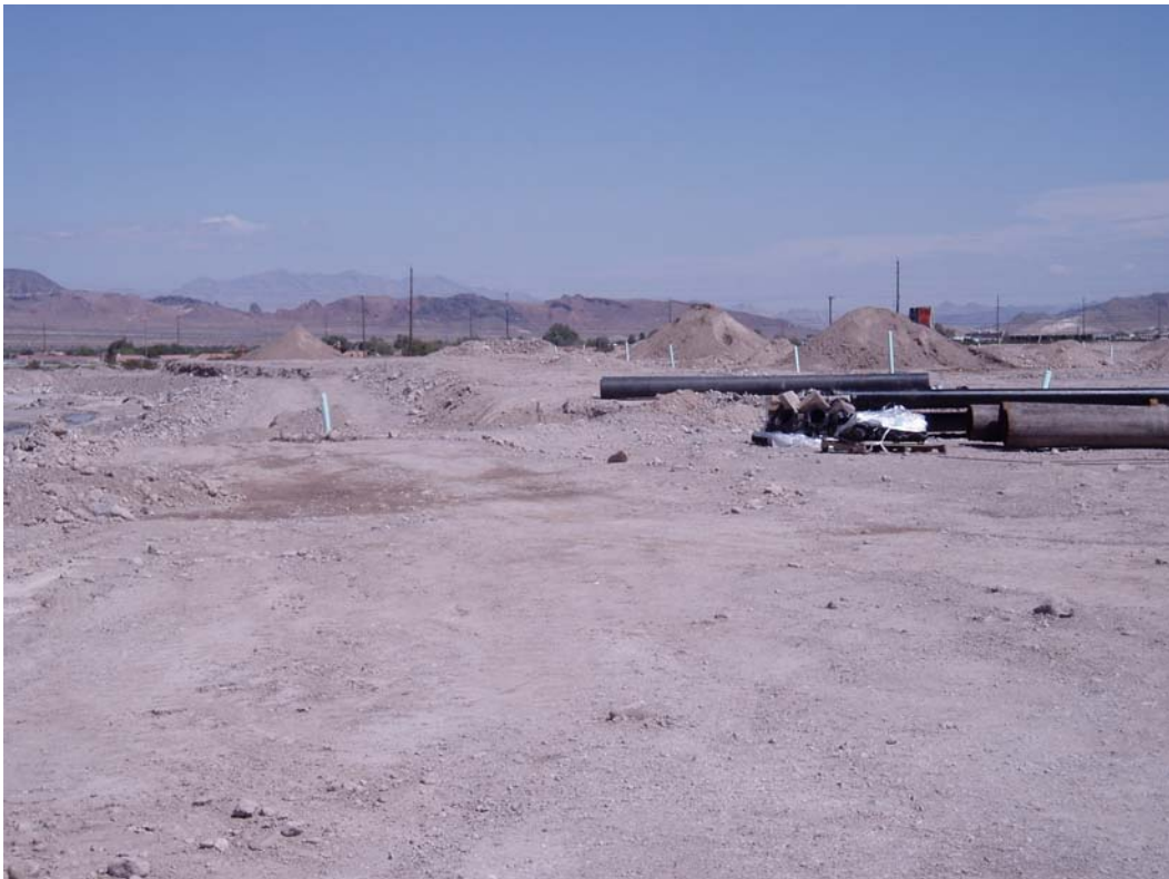
Photo 26. Construction and sediment piles (photo right) adjacent to Gibson Channel (photo left).
