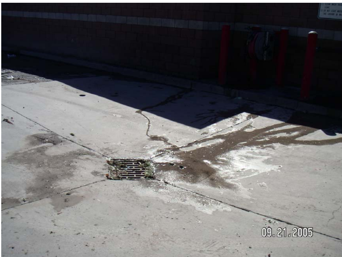
Photo 10. Grate over sand/oil interceptor.
