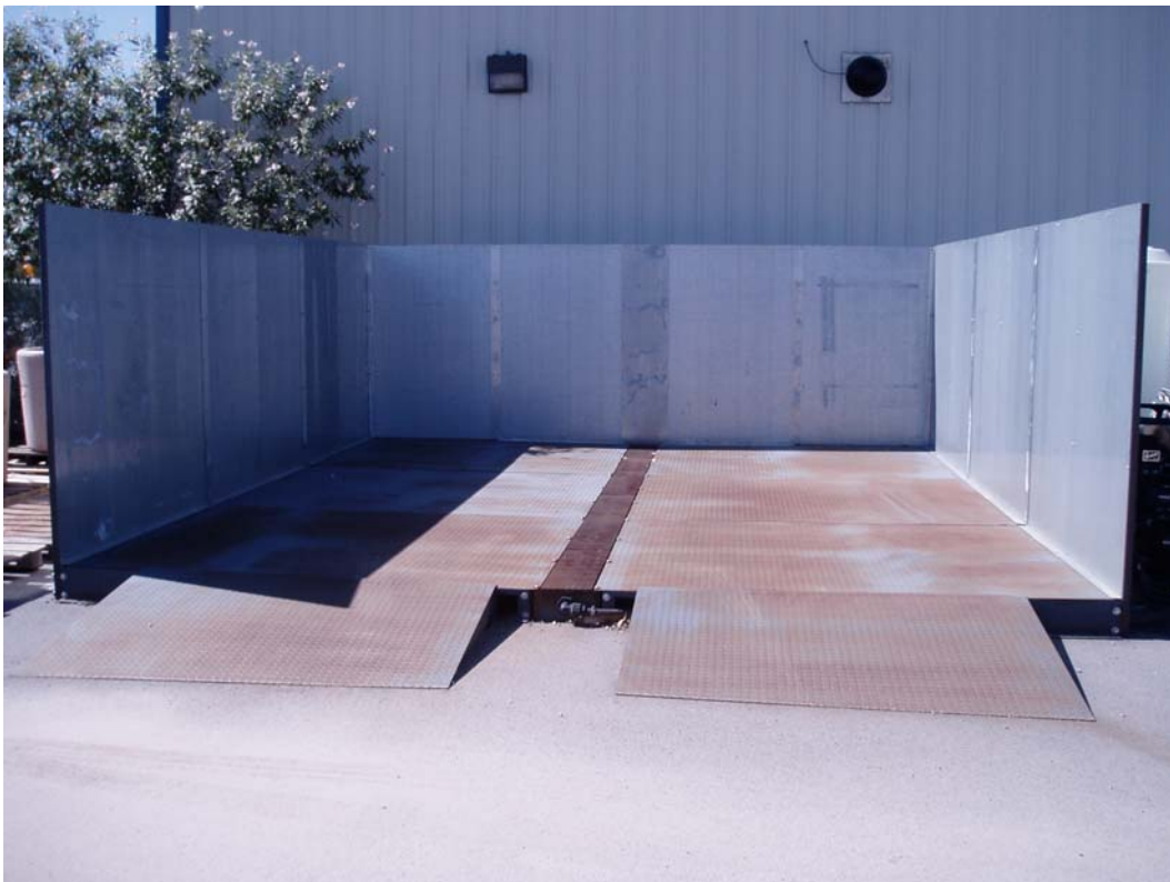
Photo 2. Equipment wash area with water recycling unit.
