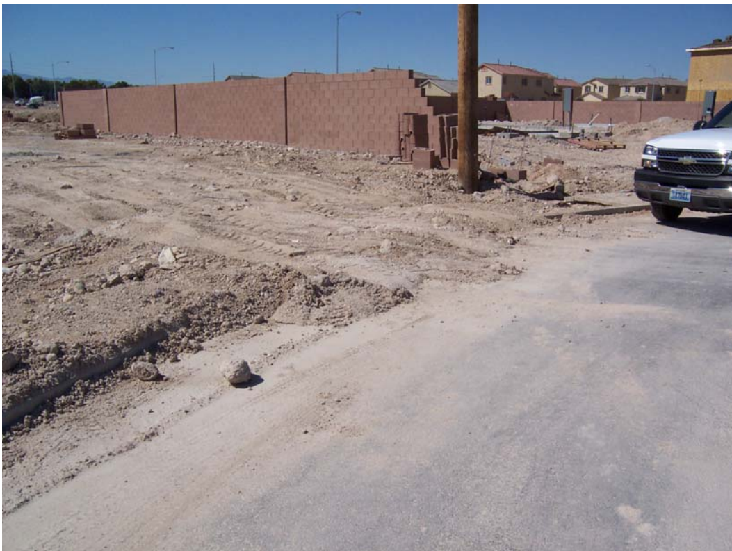
Photo 6. Absence of trackout controls at a site entrance. Note dirt extended past curb line into the street.
