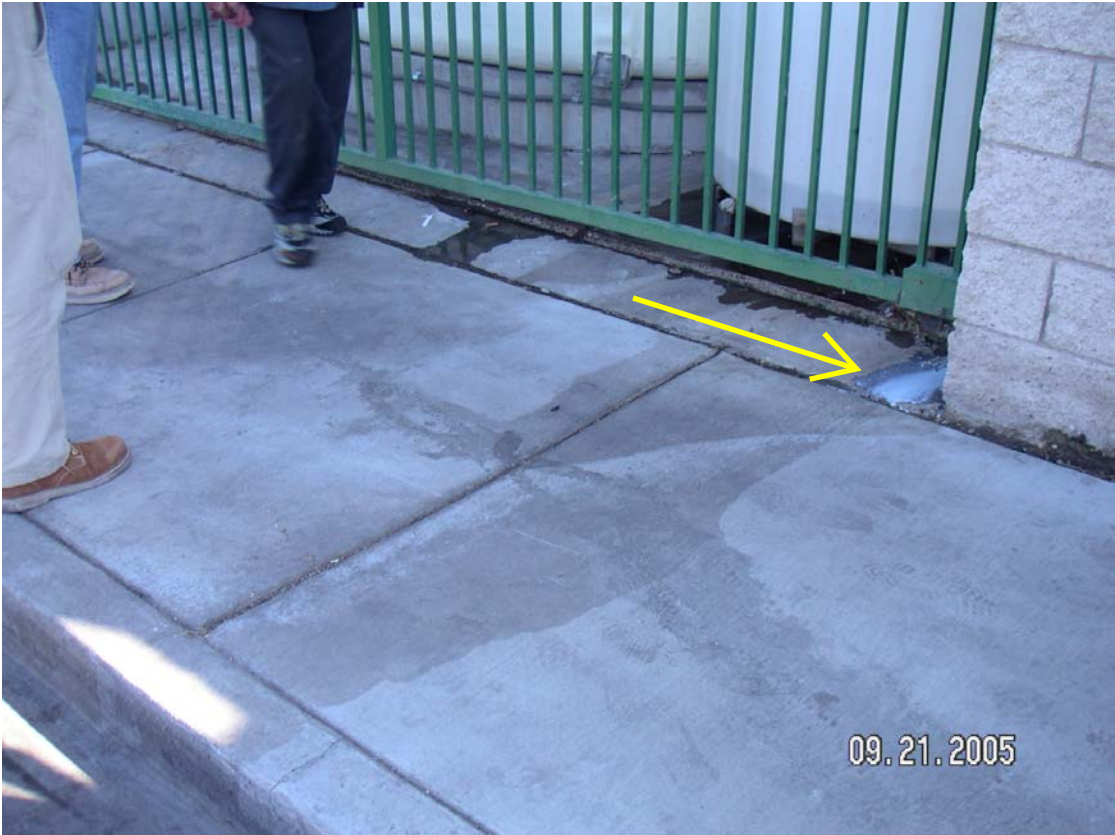
Photo 9. Discharge to street from leaking tank.
