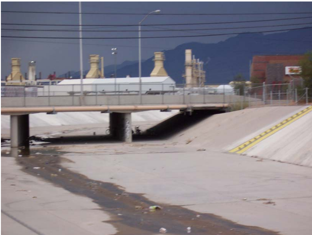
Photo 2. Loss Road overpass across the wash. Las Vegas Cogeneration facility is in the background.
