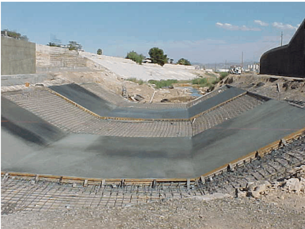
Photo 4. View downstream from earthen dam of Duck Creek Channel (photo center) and retaining walls (photo left and right).
