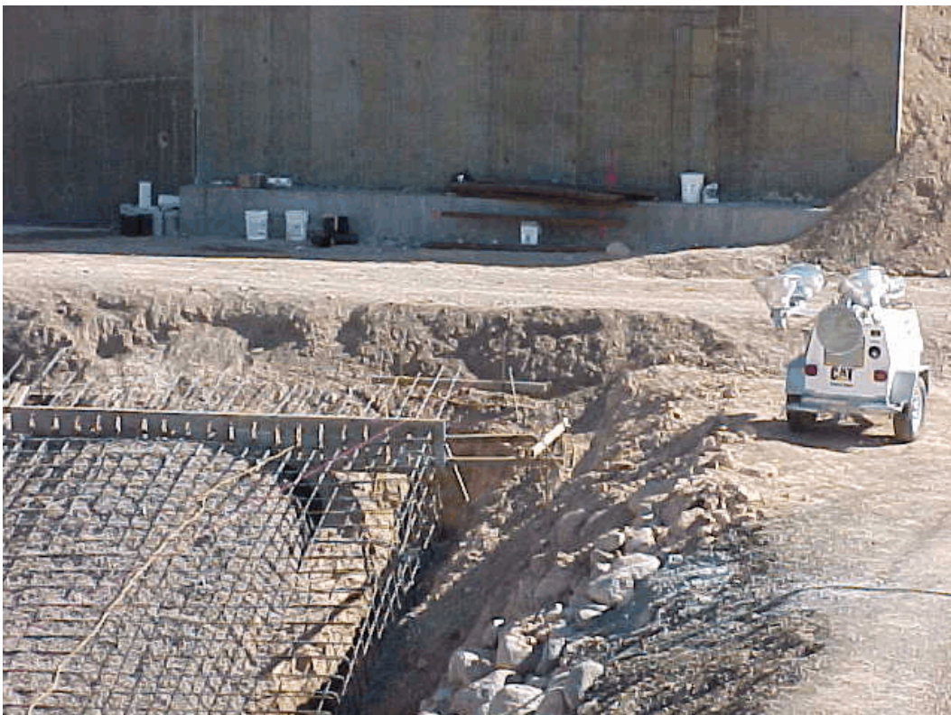
Photo 2. Downstream side of earthen dam. Note concrete runoff on face of dam. Note 5-gallon pails of chemicals along the retaining wall.
