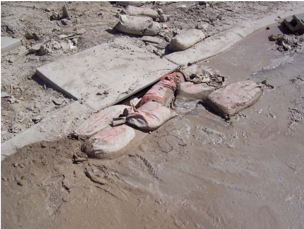
Photo 3. Different storm inlet at the site. Separation between sand bag at the right and curb allows sediment to enter the inlet.
