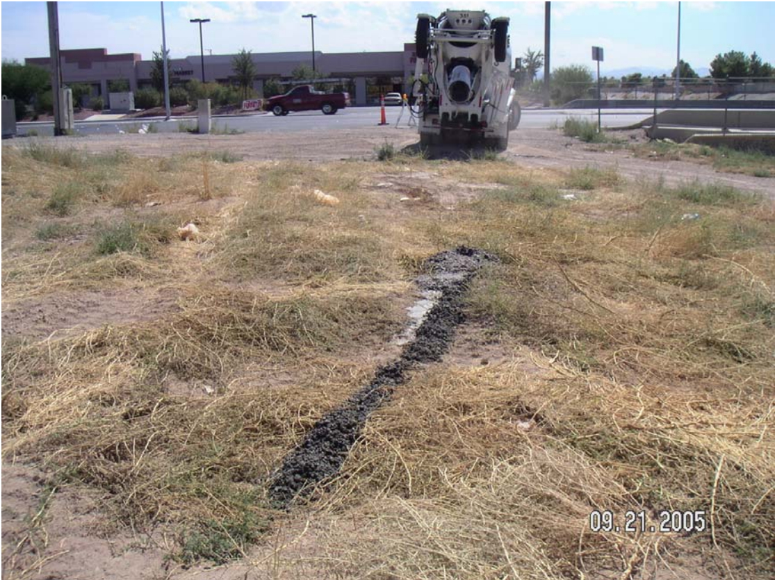
Photo 2. Wash-out material left by concrete truck.
