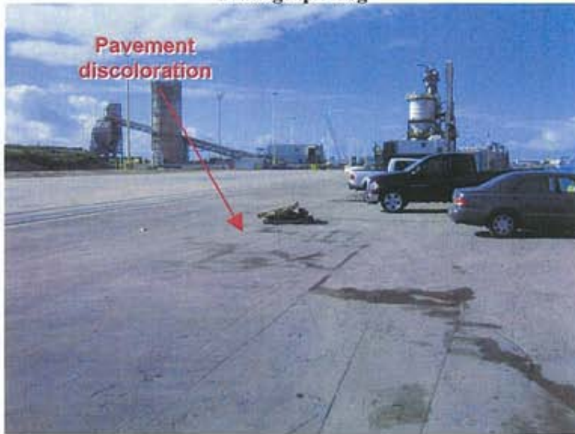
Photograph 13: Pavement discoloration and/or spill residues near the crane site
