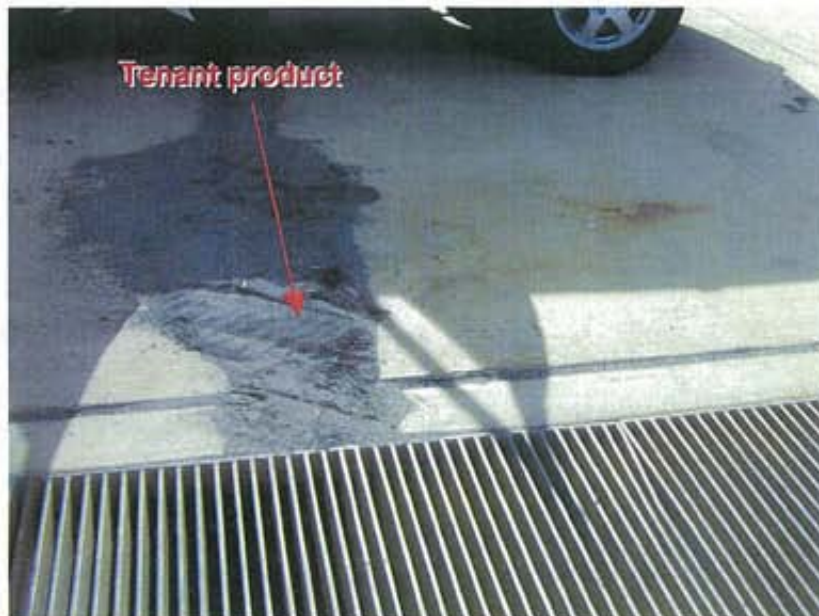
Photograph 22: View of spilled tenant product to the southeast of Photograph 21
