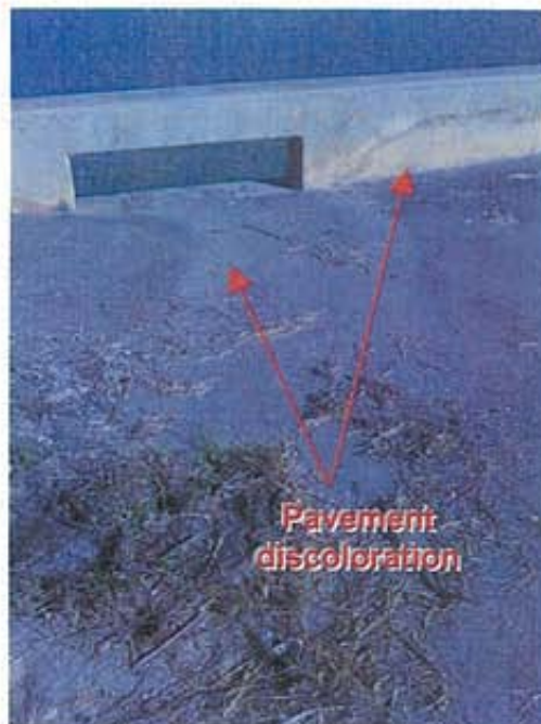
Photograph 16: Close-up view of pavement discoloration at the trench drain outlet
