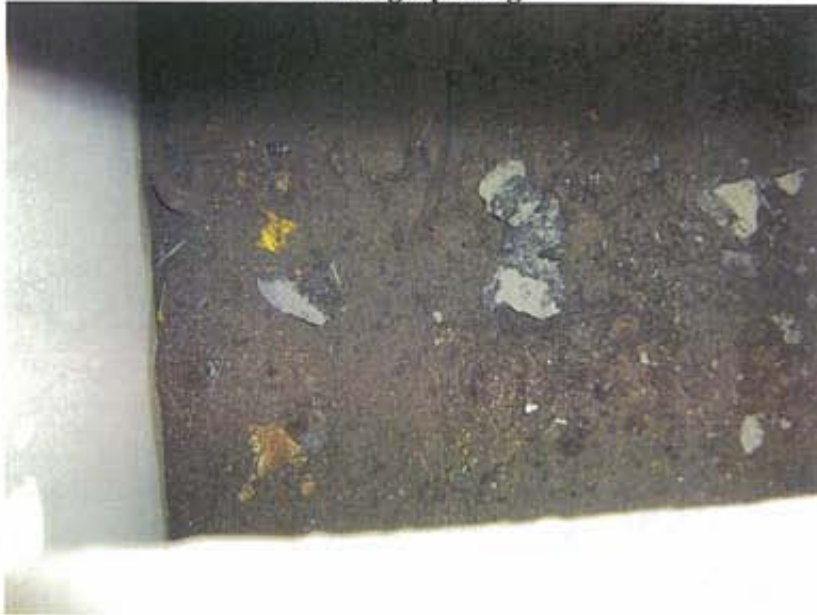
Photograph 11: Close-up view of pollutant accumulation inside the trench drain
