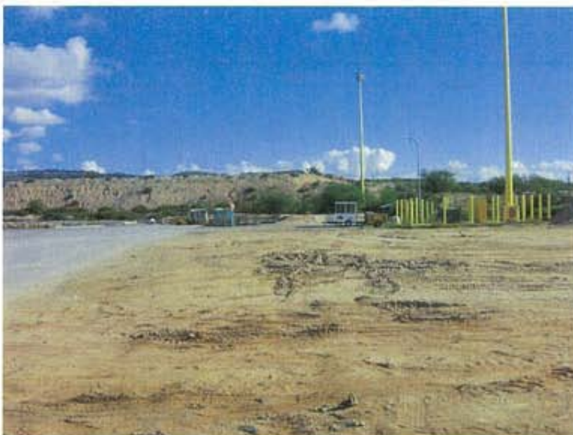
Photograph 6: View of Pier 7 showing a portion of the disturbed area associated with lighting improvements (looking northeast)
