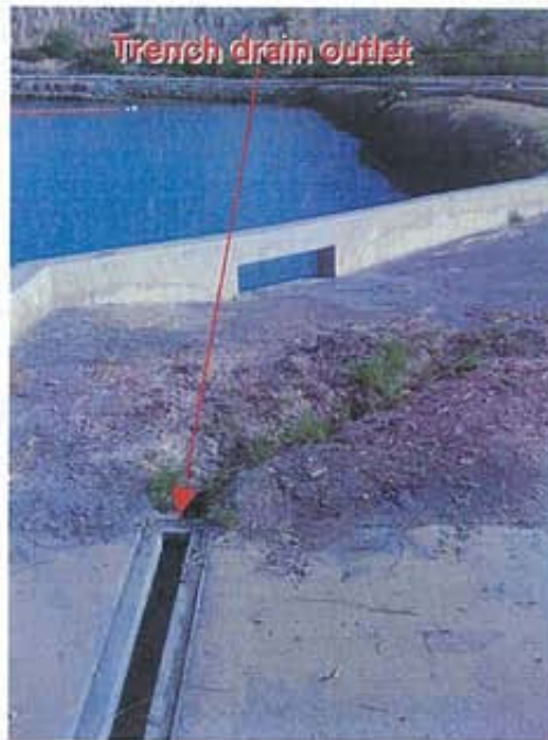
Photograph 15: Trench drain outlet and scouring at the northeast corner of Pier P-7
