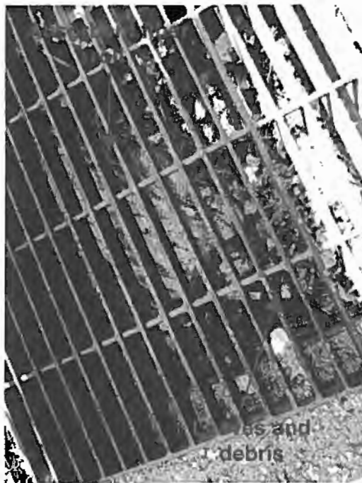
Photograph 6. Bill's Quality Auto Care – Close-up view inside the storm drain inlet shown in Photograph 5. Note that an absorbent fiber roll BMP had been placed in a drain to prevent further conveyance of petroleum to the site outfall. In addition there were leaves and debris within the catch basin.
