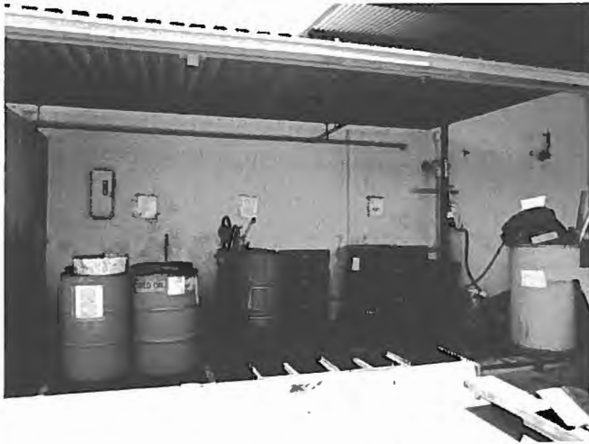
Photograph 5. Poly-Tainer, Inc. – View of the hazardous materials and hazardous waste covered storage area located on the south side of the facility building.
