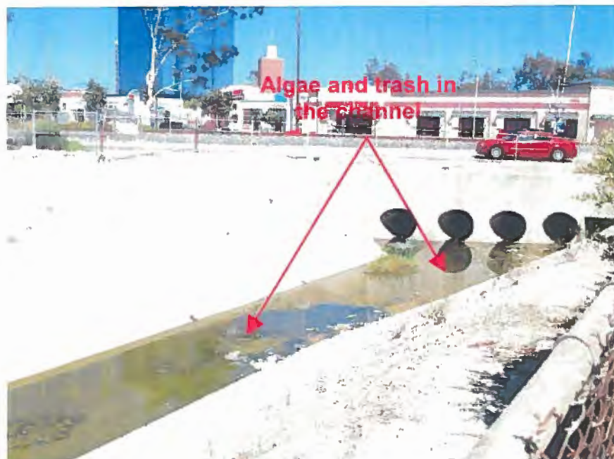
Photograph 1. City MS4 Outfall – El Rio Drain Outfall – View of the outfall from the City MS4 to the VCWPD. Note the algal growth and trash in the channel.
