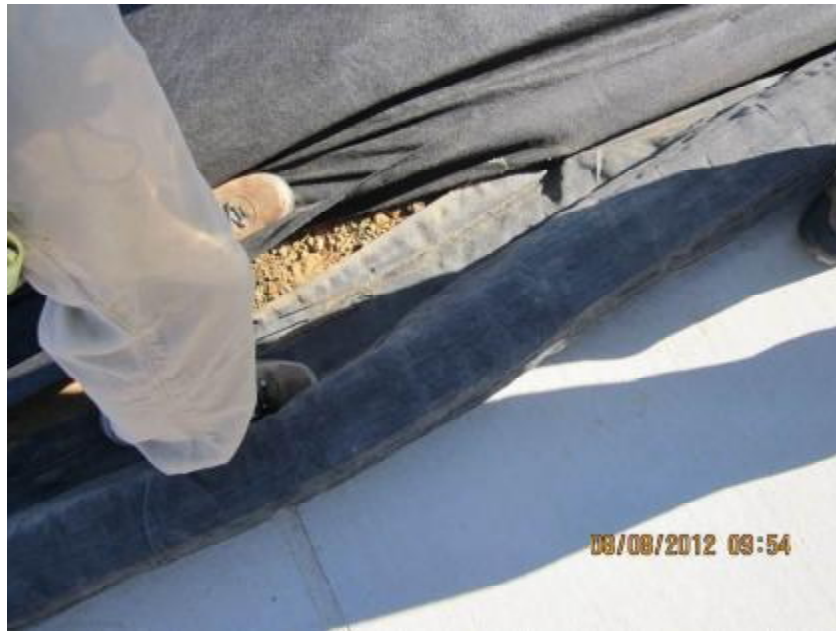
Photograph 2. View of "heavy weight wattle" sediment control BMP which was not entrenched into the ground.
