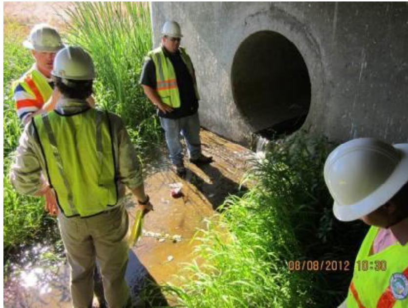
Photograph 3. View of outfall to Shed B Channel. Note dry weather flow from outfall.
