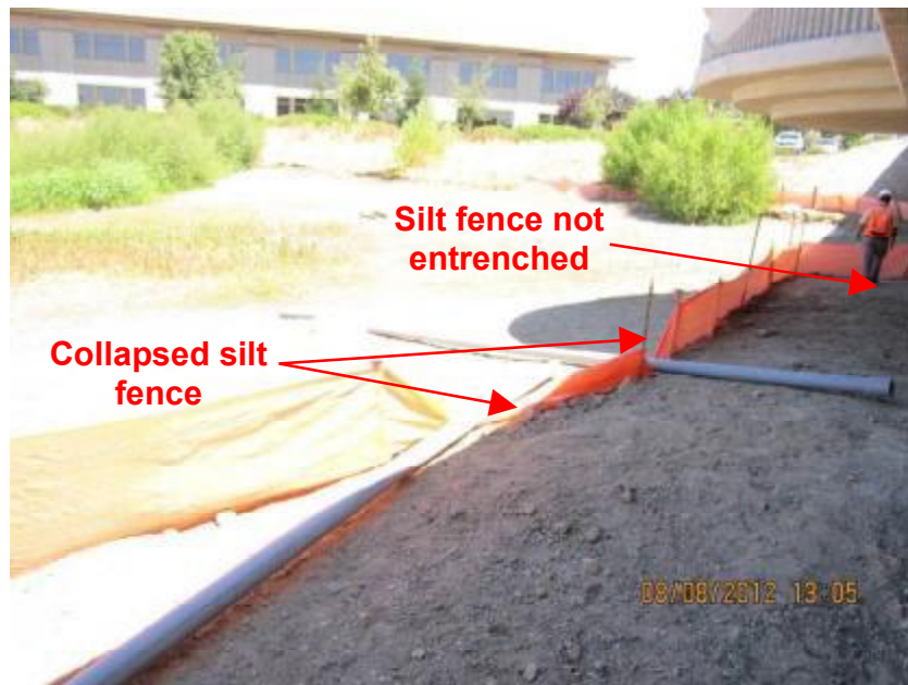
Photograph 1. Longleaf Drive Bridge Construction Project – View of area below the bridge where there was a section of collapsed silt fence and a section of silt fence that was not entrenched into the ground.
