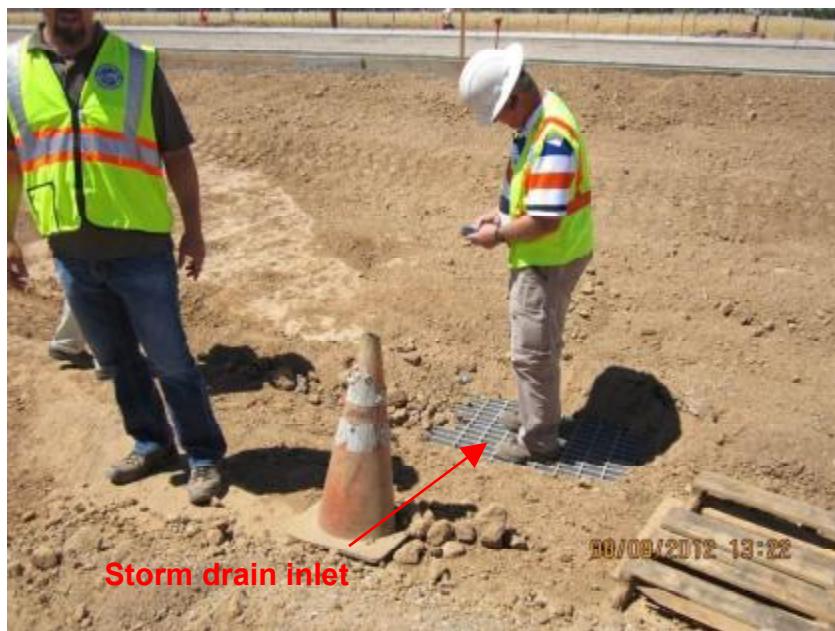
Photograph 6. Laguna Corporate Center Construction Project – View of storm drain inlet without inlet protection along south side of the roadway extension construction from the bridge.
