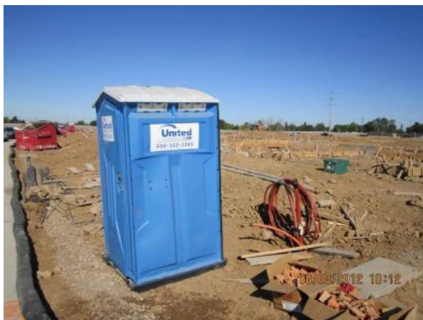
Photograph 4. View of an additional portable toilet at the site which was not staked into the ground or otherwise secured.
