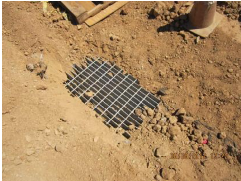
Photograph 7. Laguna Corporate Center Construction Project – Close-up view of storm drain inlet shown in Photograph 6.
