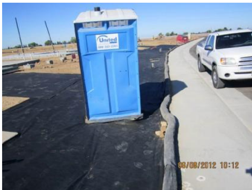
Photograph 3. View of portable toilet at the site which was not staked into the ground or otherwise secured.
