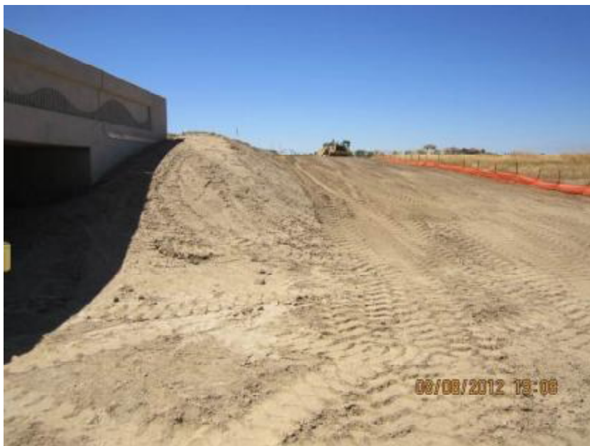
Photograph 5. Longleaf Drive Bridge Construction Project – View of north abutment on west side of the bridge. Note lack of erosion and sediment control BMPs.
