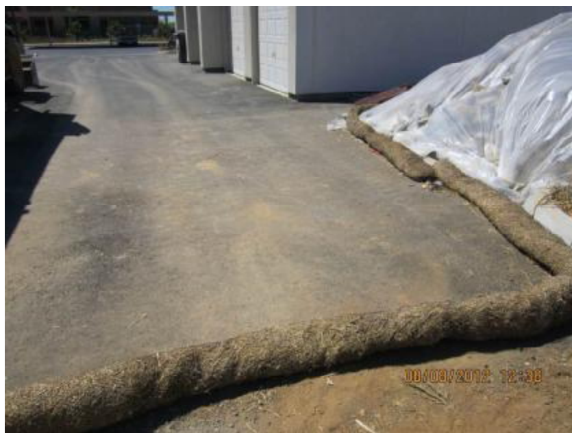
Photograph 4. Additional example of stockpile surrounded by straw wattles which were not entrenched into the ground.
