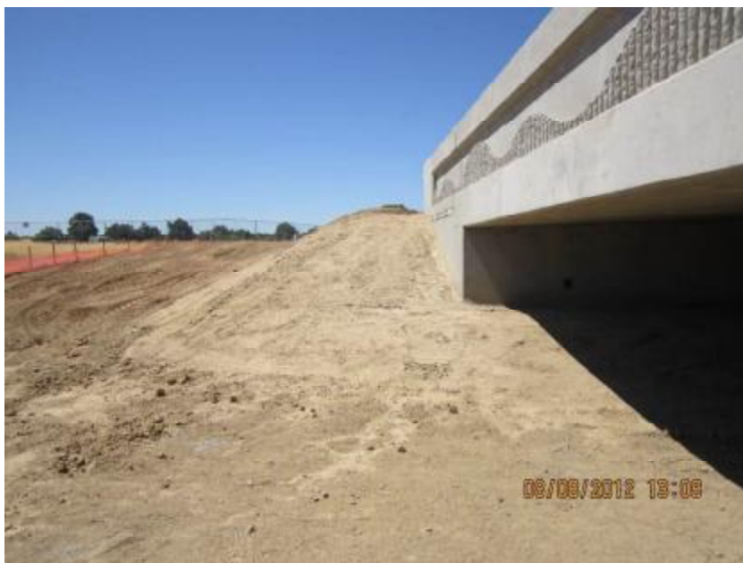
Photograph 4. Longleaf Drive Bridge Construction Project – View of south abutment on west side of the bridge. Note lack of erosion and sediment control BMPs.
