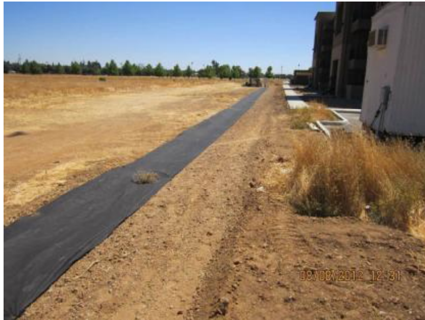
Photograph 1. View looking east of northern perimeter of the construction site. Note that BMPs had not been installed for perimeter control.
