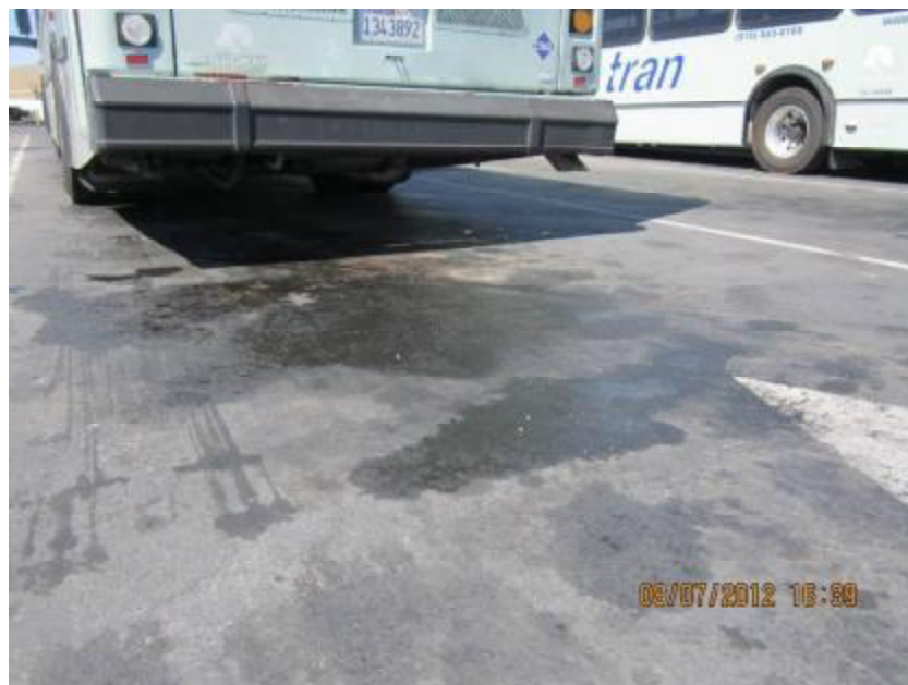
Photograph 10. Closer view of staining shown in Photograph 9.
