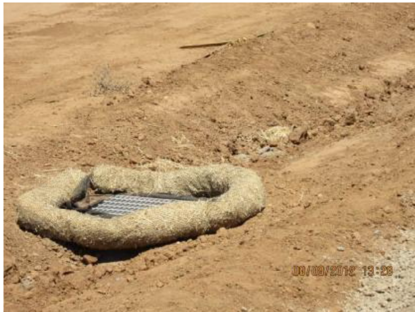
Photograph 8. Laguna Corporate Center Construction Project – View of storm drain inlet in parking lot area surrounded by straw wattles which were not entrenched into the ground.
