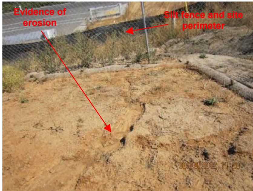
Photograph 5. View of straw wattle BMPs and silt fence BMP installed near the northeast corner of the site. Note evidence of erosion in foreground of the photograph.
