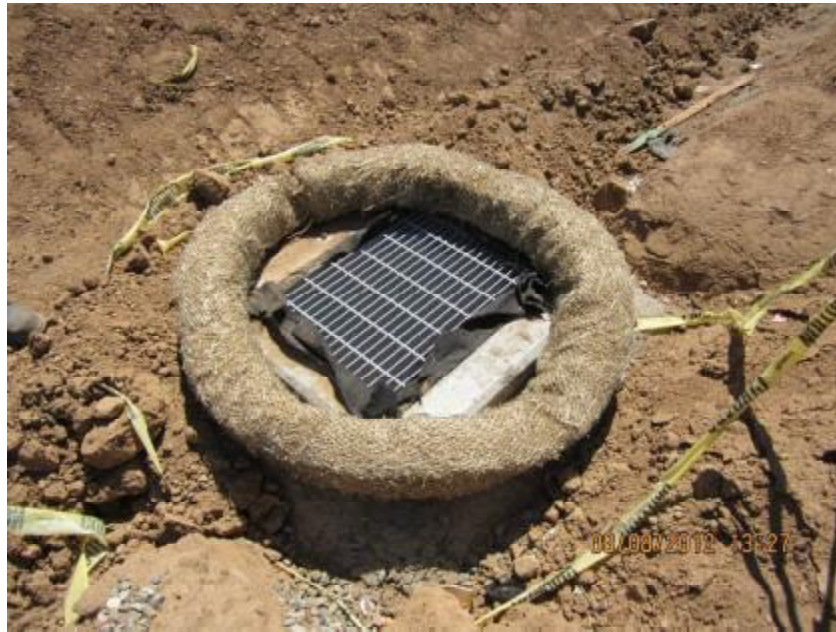
Photograph 9. Laguna Corporate Center Construction Project – Additional example of storm drain inlet in parking lot area surrounded by straw wattles which were not entrenched into the ground.
