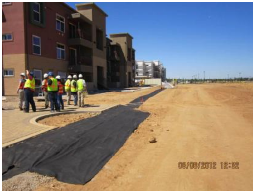
Photograph 2. View looking west of northern perimeter of the construction site. Note that BMPs had not been installed for perimeter control.
