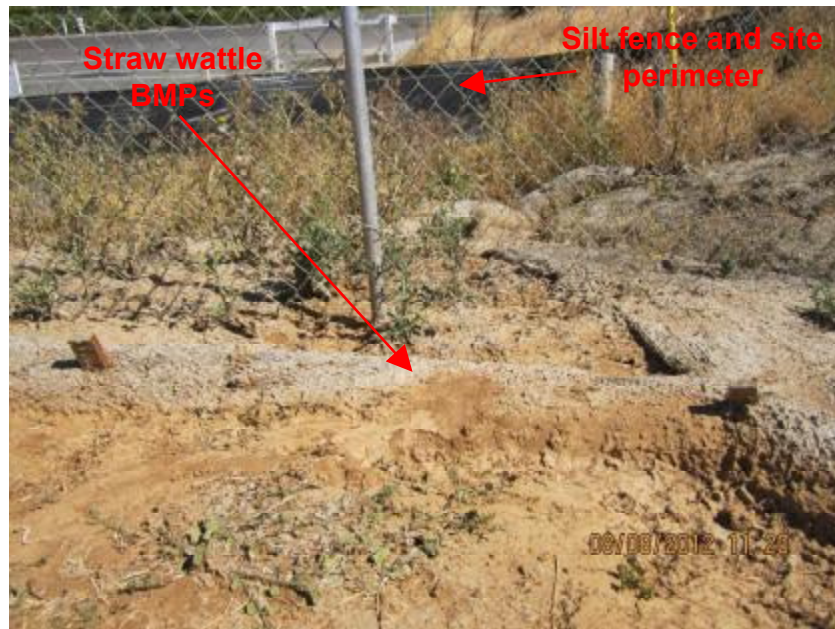
Photograph 6. Close-up view of straw wattle which had accumulated sediment to its full height.
