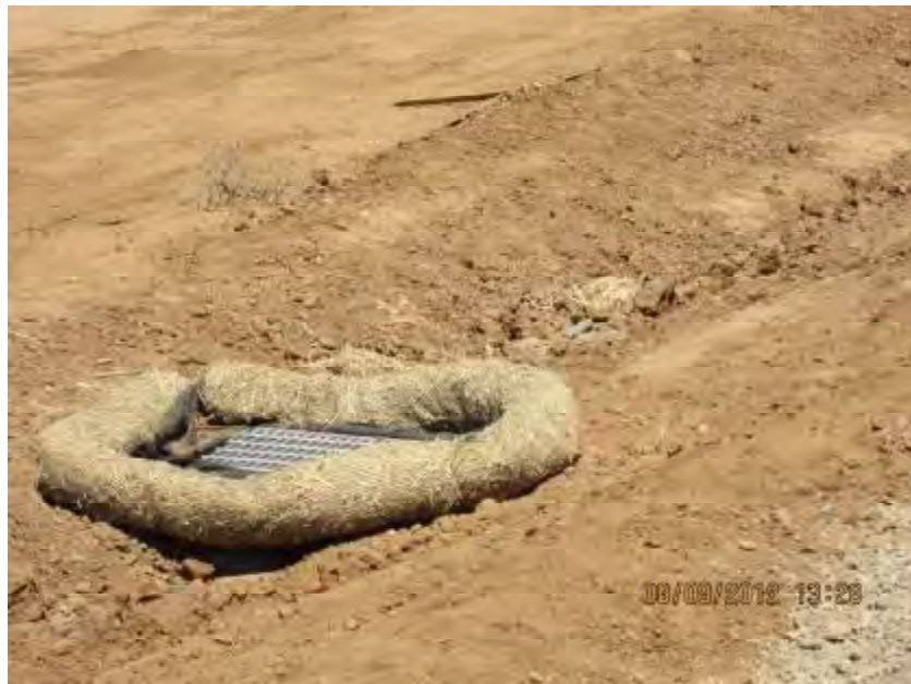
Photograph 8. Laguna Corporate Center Construction Project – View of storm drain inlet in parking lot area surrounded by straw wattles which were not entrenched into the ground.
