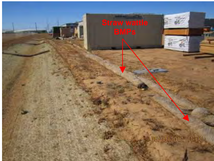
Photograph 3. View of straw wattle BMPs installed along the eastern edge of the site. Note that the straw wattles were not entrenched into the ground.
