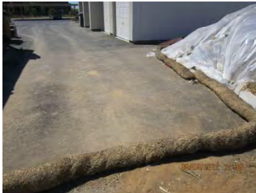
Photograph 4. Additional example of stockpile surrounded by straw wattles which were not entrenched into the ground.
