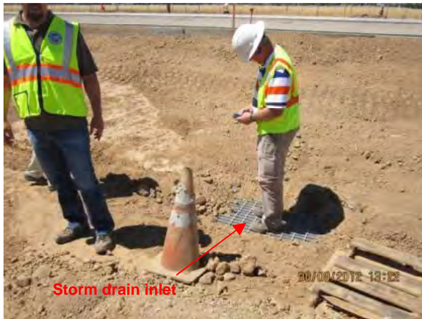
Photograph 6. Laguna Corporate Center Construction Project – View of storm drain inlet without inlet protection along south side of the roadway extension construction from the bridge.
