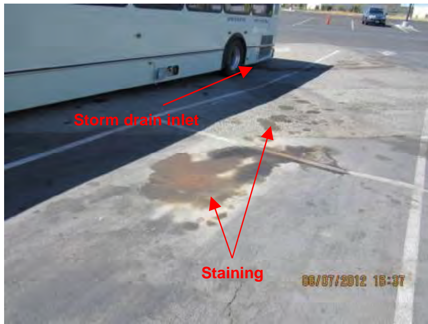
Photograph 8. View of staining on pervious and impervious ground surface upgradient of storm drain inlet shown in Photographs 6 and 7.
