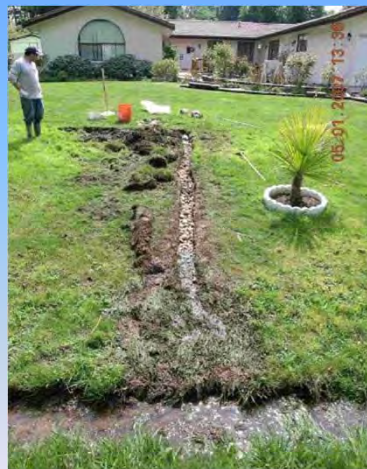
Illicit Discharge of Sewage from Failing Septic System Drain field
