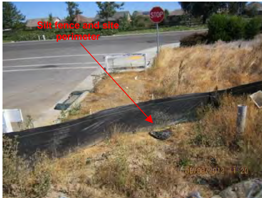
Photograph 7. View of silt fence BMP installed downgradient of the straw wattles shown in Photographs 5 and 6.
