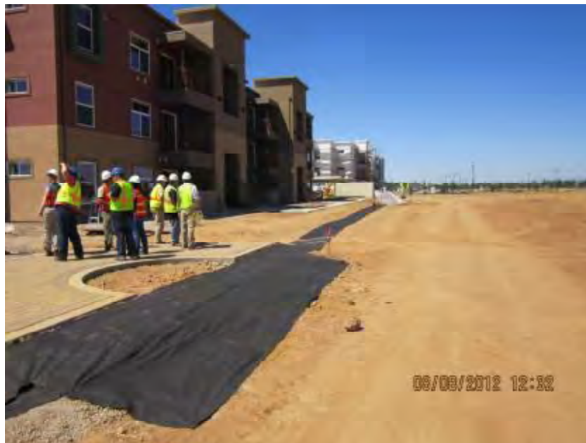
Photograph 2. View looking west of northern perimeter of the construction site. Note that BMPs had not been installed for perimeter control.
