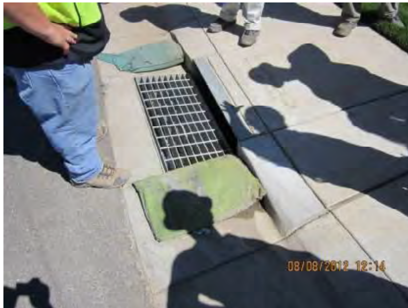
Photograph 4. View of deteriorated gravel bags used for storm drain inlet protection.
