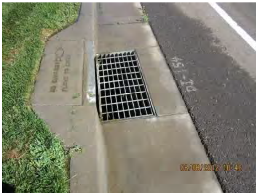
Photograph 6. Close-up view of storm drain inlet noted in Photograph 5. Note wetted area surrounding inlet.
