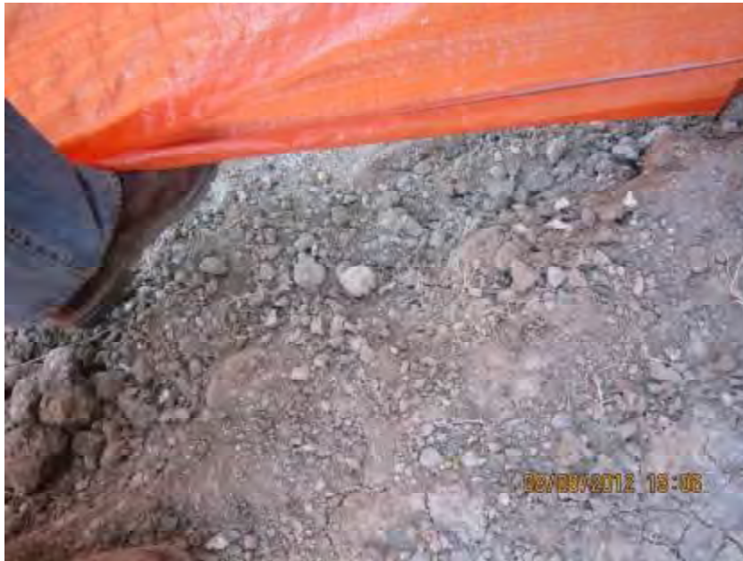
Photograph 3. Longleaf Drive Bridge Construction Project – Additional view of silt fence shown in Photographs 1 and 2 that was not entrenched into the ground.
