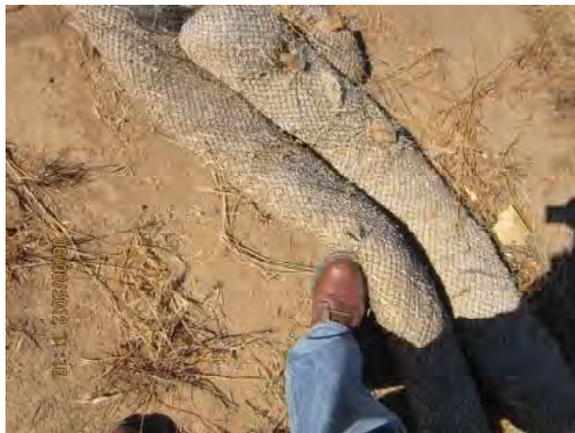
Photograph 4. Close-up view of straw wattles along the eastern edge of the site which were not entrenched into the ground.
