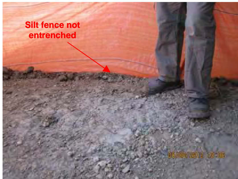
Photograph 2. Longleaf Drive Bridge Construction Project – Closer view of section of silt fence that was not entrenched into the ground noted in Photograph 1.
