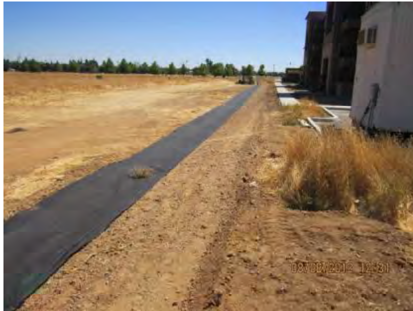
Photograph 1. View looking east of northern perimeter of the construction site. Note that BMPs had not been installed for perimeter control.
