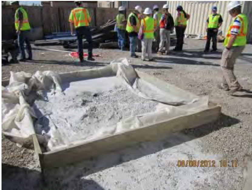
Photograph 5. View of concrete washout area at the site. Note concrete waste material located adjacent to the washout containment structure.
