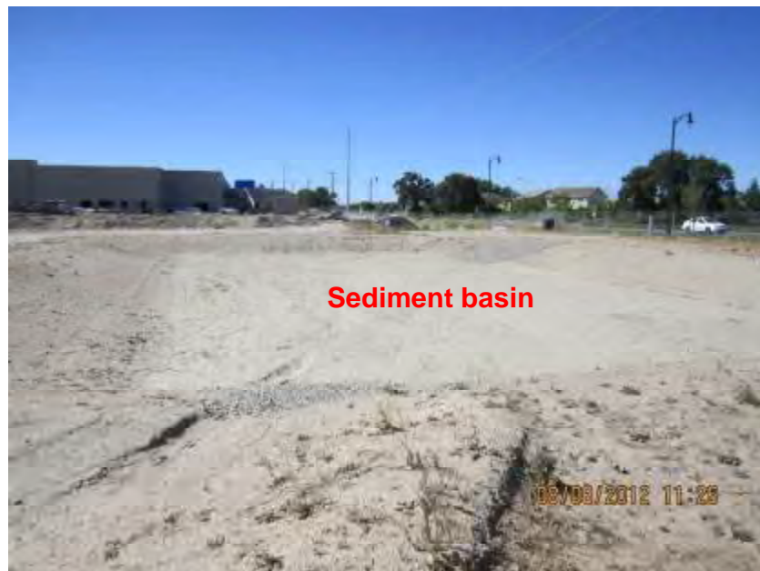
Photograph 2. View of temporary sediment basin near the northwest corner of the site.
