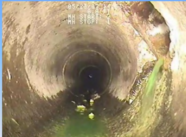
Illicit Connection identified by CCTV cameras
