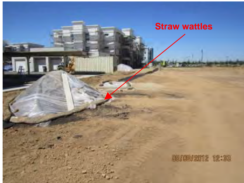
Photograph 3. View of stockpile along northern perimeter of the construction site. Note that the straw wattles placed around the stockpile were not entrenched into the ground.
