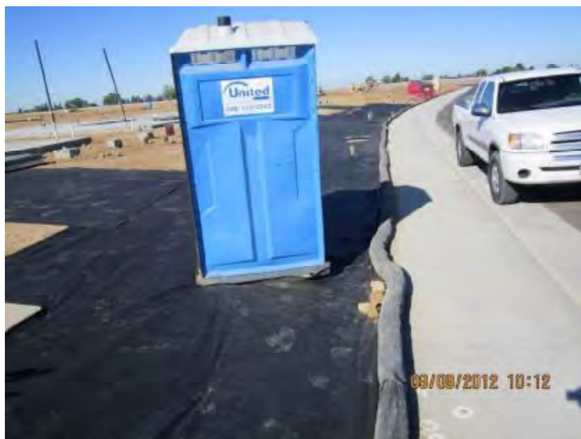
Photograph 3. View of portable toilet at the site which was not staked into the ground or otherwise secured.
