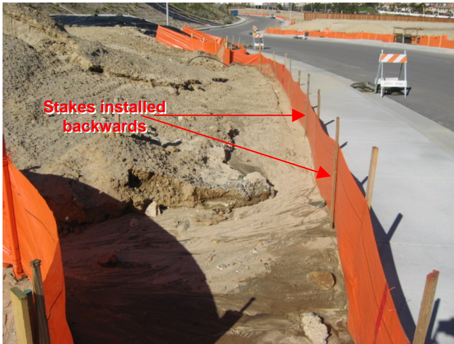
Photograph 8: The silt fence was not installed on the contour and stakes were incorrectly positioned on the up-gradient side of the silt fence
