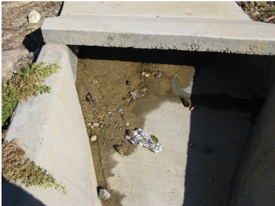
Photograph 10: Sediment accumulated in the drainage conveyance located down-gradient of Photographs 8 and 9
