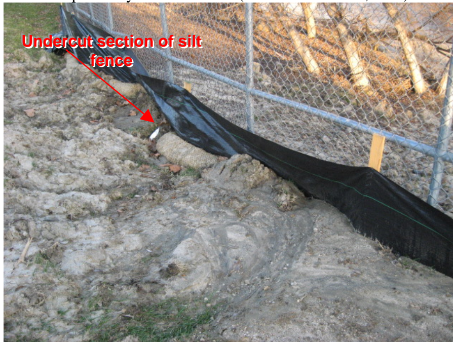
Photograph 3: A section of silt fence at the base of the slope had been undercut by a previous flow event
