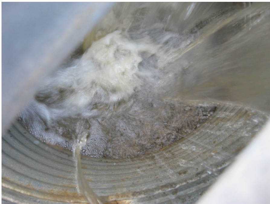
Photograph 16: View inside storm drain inlet leading to the Pechanga Parkway Drainage Channel
