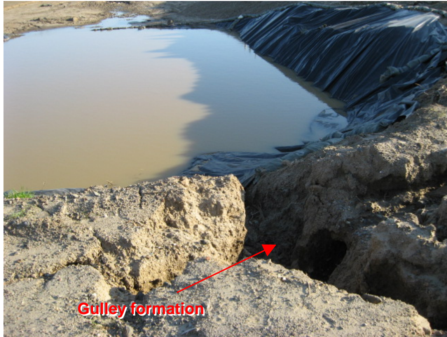
Photograph 5: Sediment laden water in the structural control and gulley erosion present at the inlet area
