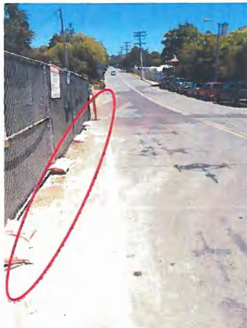
Photograph 2. Many Mansions Site Visit – View facing east on Los Feliz Drive of unstablized soil outside the perimeter construction fence.
