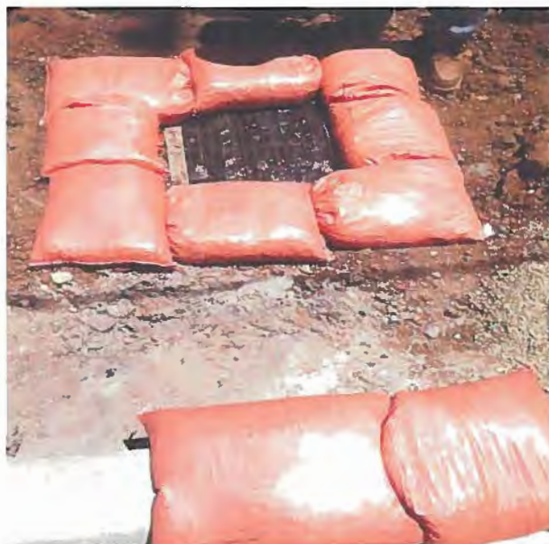
Photograph 9. Many Mansions Site Visit – View of grate inlet covered with geotextile and sand bags placed around the edge of the inlet.
