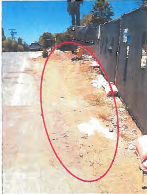
Photograph 1. Many Mansions Site Visit – View facing west on Los Feliz Drive of unstablized soil outside the perimeter construction fence.
