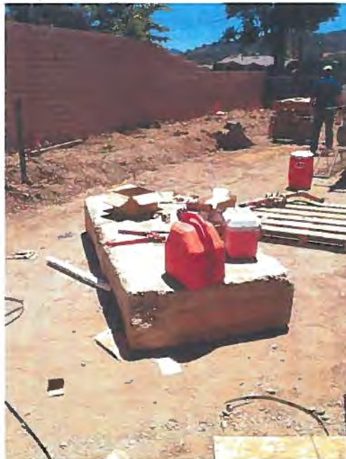
Photograph 6. Many Mansions Site Visit – View of gasoline container without secondary containment.
