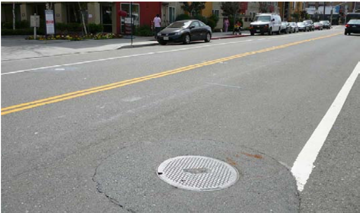
Emeryville Photo 6: 1400 65th Street - manhole cover showing pickhole that wastewater came out of.
