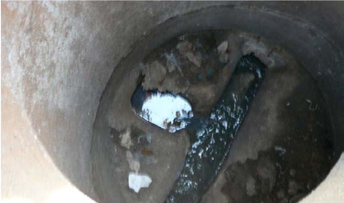
Emeryville Photo 5: Manhole outside 1400 65th Street, where grease blockage occurred.
