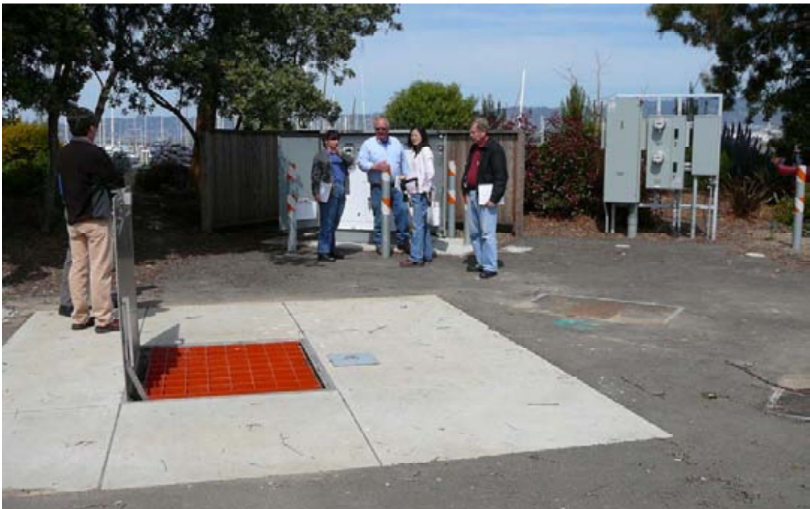
Emeryville Photo 4: Marina pump station and controller box.
