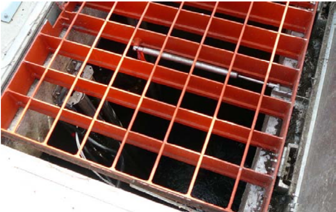
Emeryville Photo 2: Safety cover over Marina pump station wet well.
