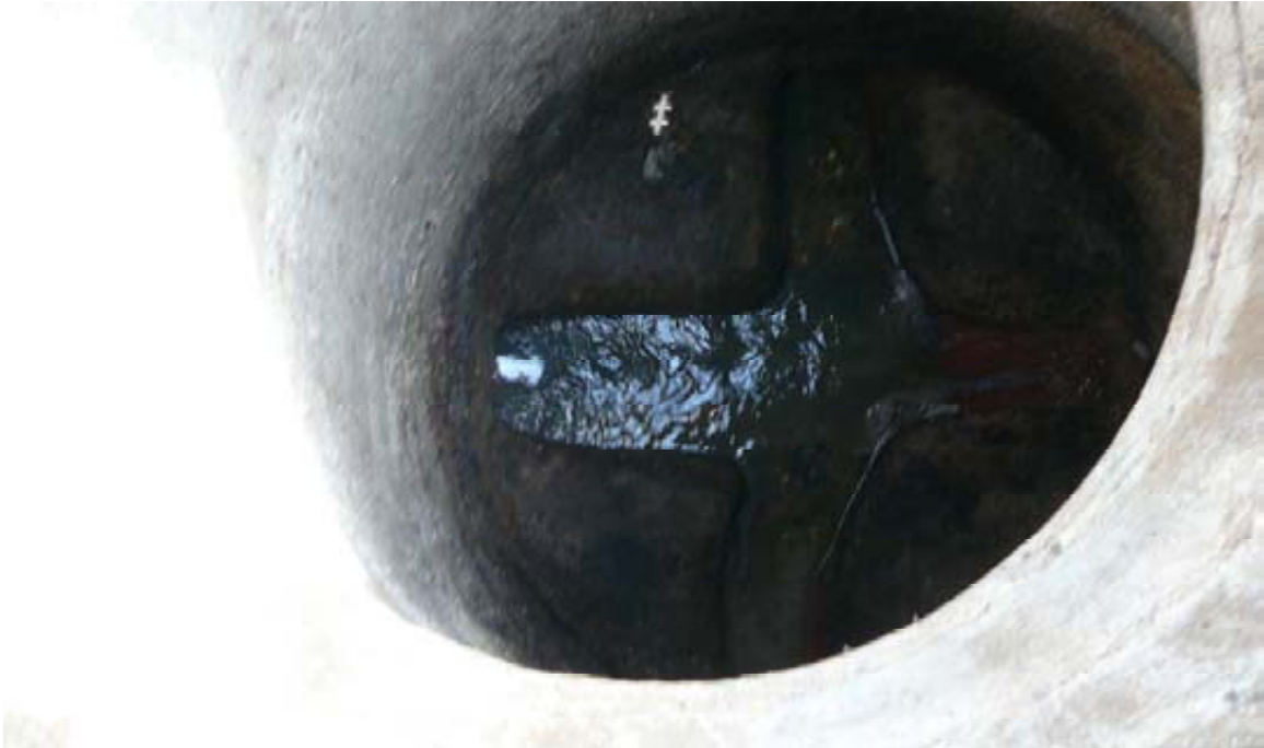
Emeryville Photo 7: Manhole that overflowed at 63rd Street due to debris. Oakland flow enters from left.
