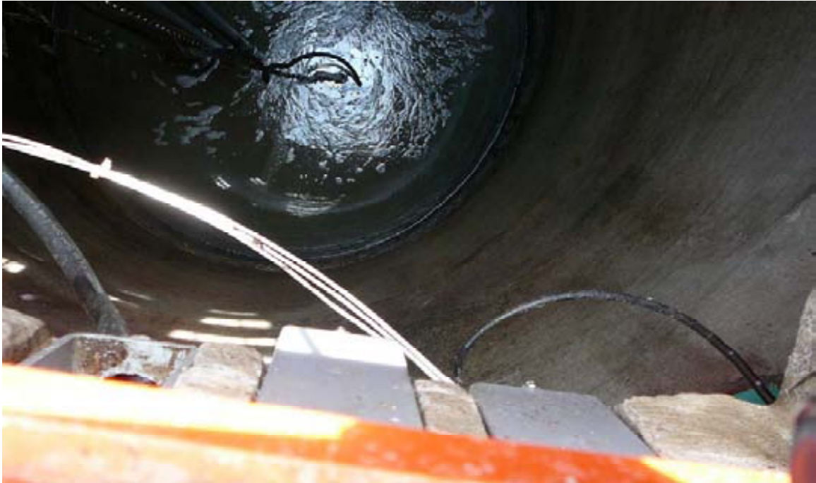
Emeryville Photo 1: Marina pump station wet well. Some grease visible.
