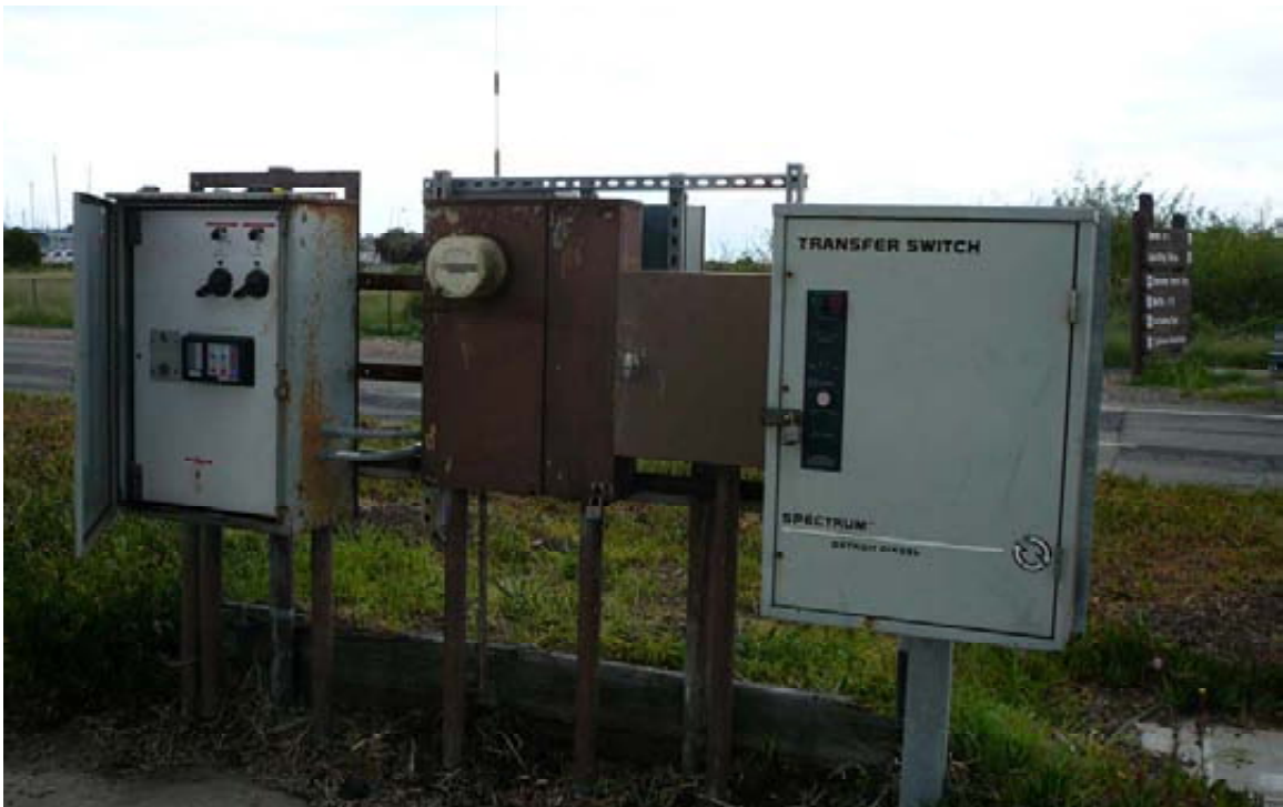
Berkeley Photo 4: Pump station 5 controls.
