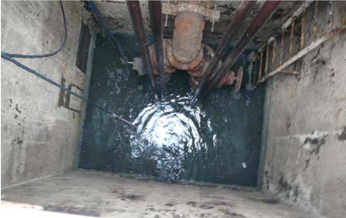
Berkeley Photo 3: Pump station 5 wet well.
