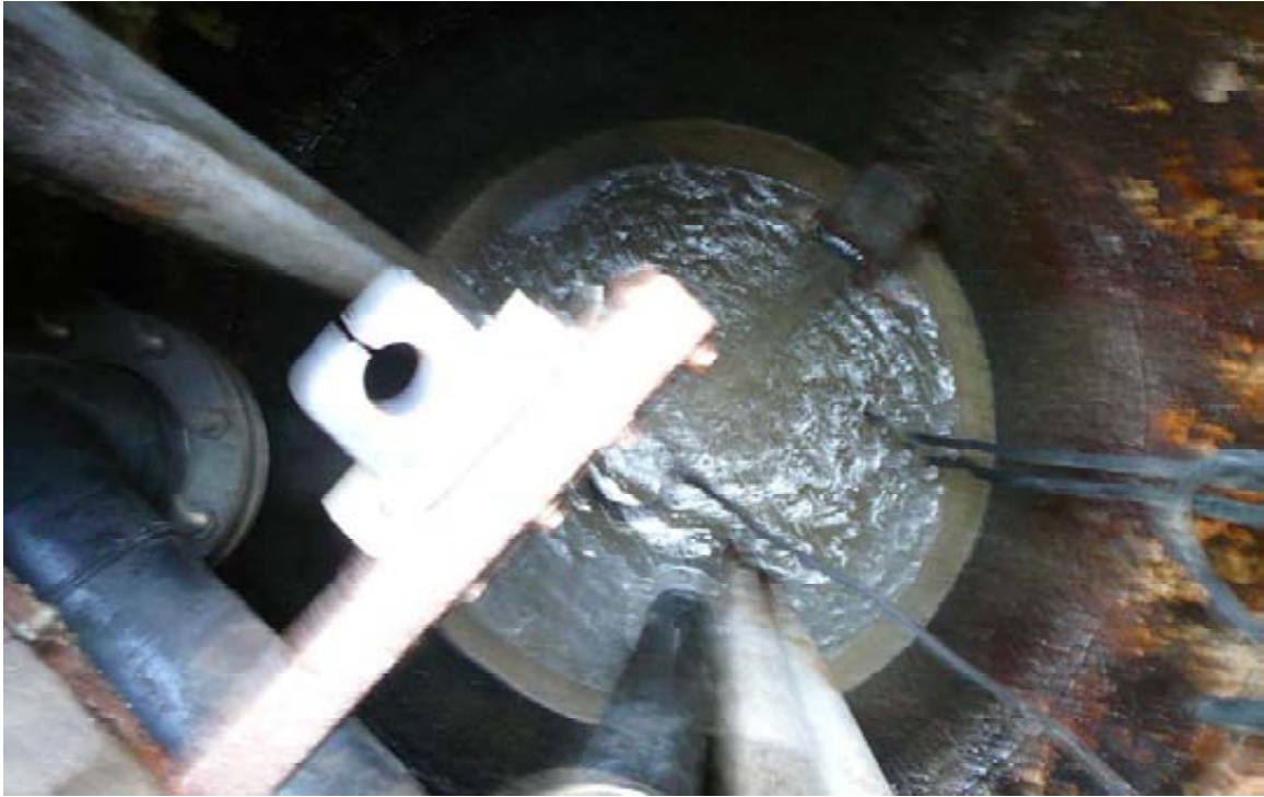
Berkeley Photo 5: Pump station 3 wet well.
