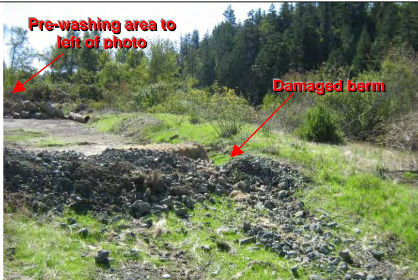
Photograph 7— Damaged berm shown in Photograph 6
