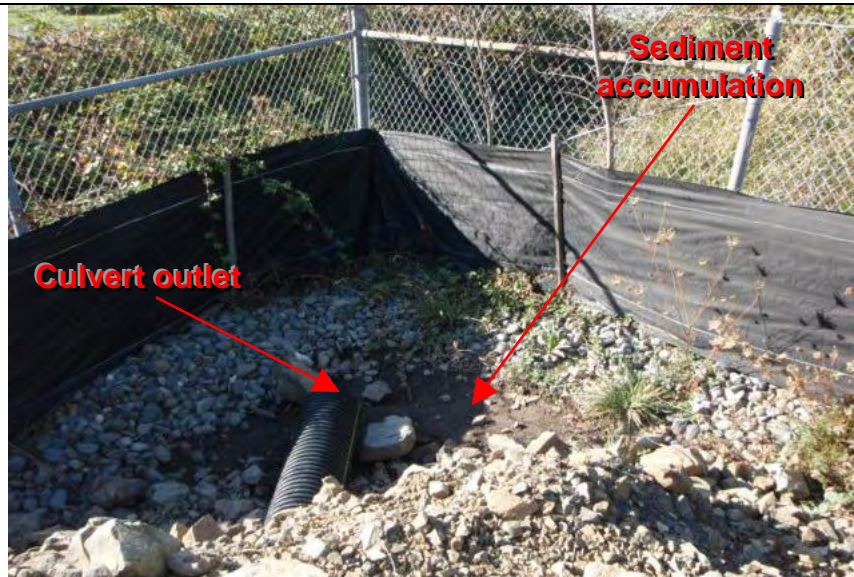
Photograph 3 – Culvert outlet to northwest corner of facility (Note: Silt fence BMP installed backwards)
