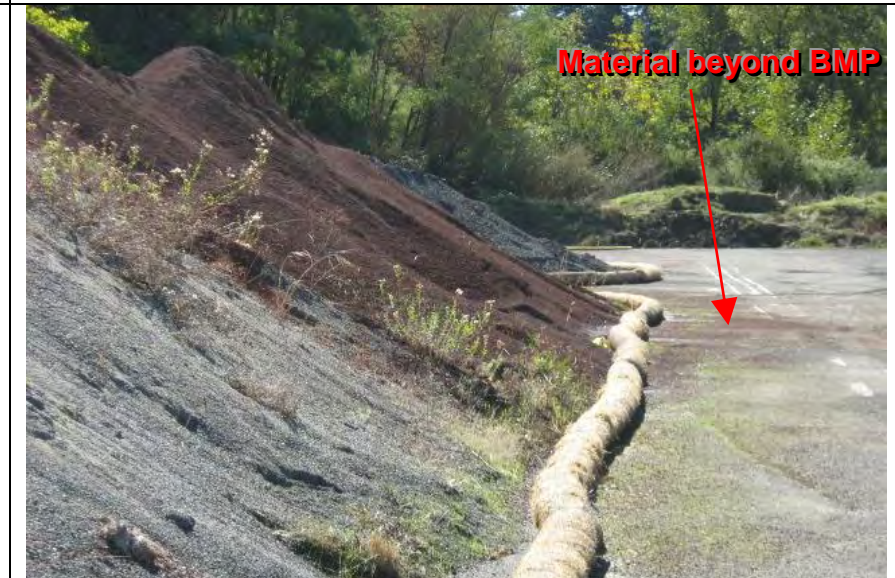
Photograph 8 – Inappropriate application of wattles on impervious surface
