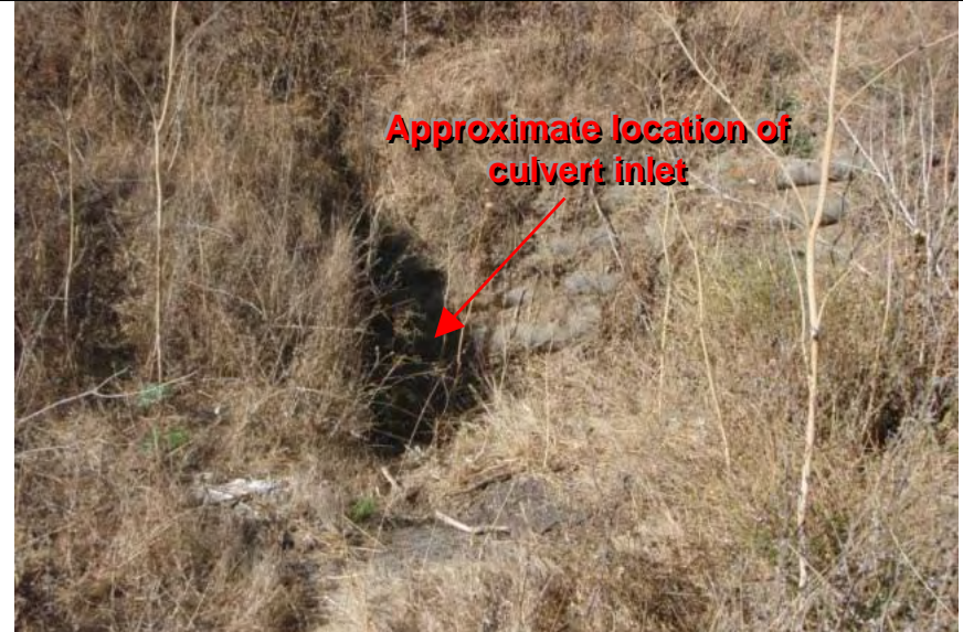
Photograph 6 – Location of culvert inlet in the northwestern portion of the waste storage site
