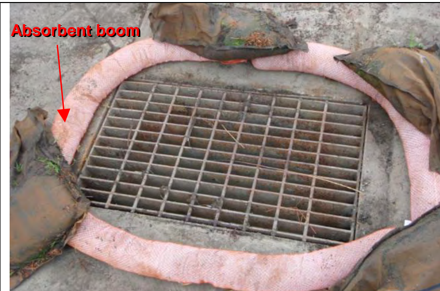
Photograph 5— Closer view of storm drain inlet shown in Photograph 3
