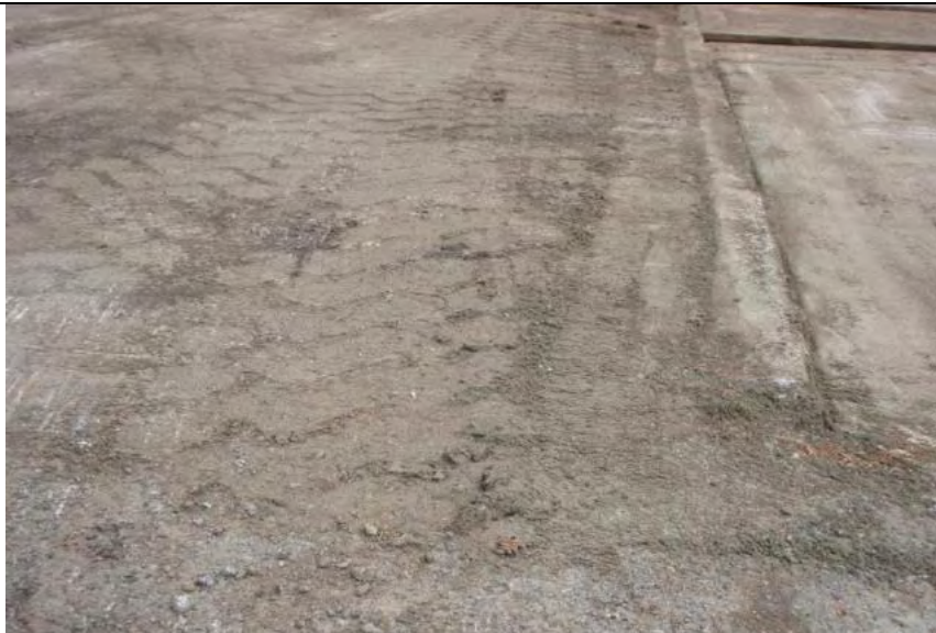
Photograph 7— Closer view of sediment accumulation on imperious ground surface
