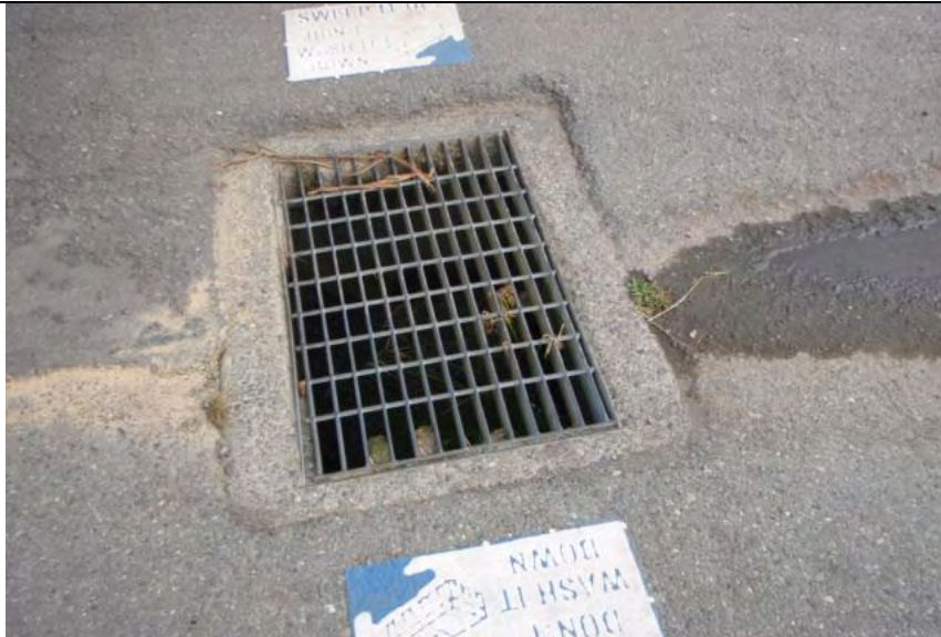
Photograph 1 – Storm drain inlet at facility
