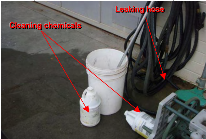
Photograph 11— Cleaning/washing chemicals stored on impervious ground surface adjacent to leaking hose
