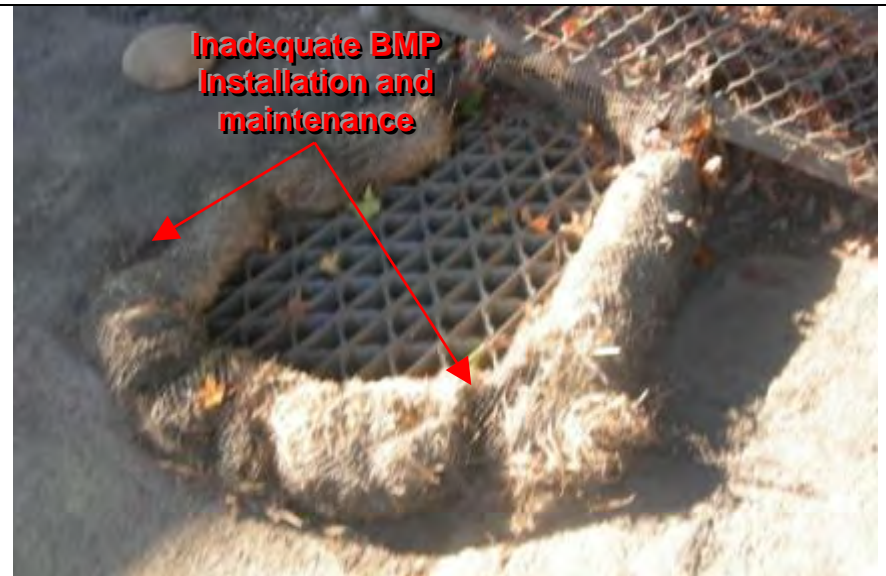
Photograph 4 – Storm drain inlet on the east side of the Marysville Maintenance Station office building
