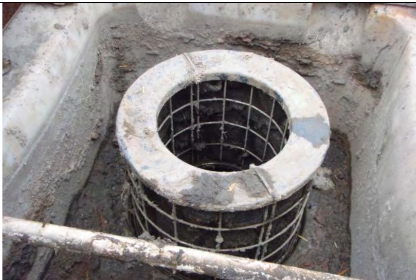
Photograph 9— Closer view of filter shown in Photograph 8. (Note: Pollutant accumulation within filter and inlet)
