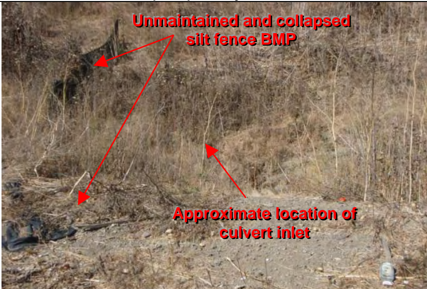
Photograph 7 – Location of culvert inlet and unmaintained and collapsed silt fence BMP up-gradient of inlet
