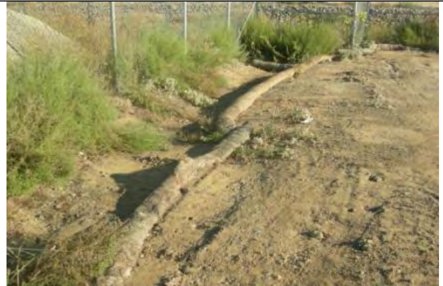
Photograph 2 – View of straw wattle BMPs, not adequately installed
