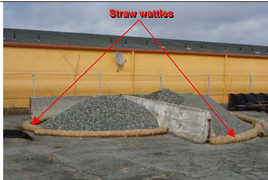
Photograph 10 – Inappropriate application of wattles on impervious surface
