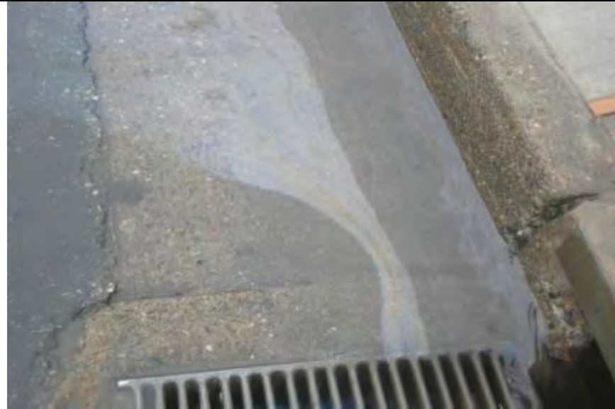
Photograph 1 – Visible sheen entering storm drain
