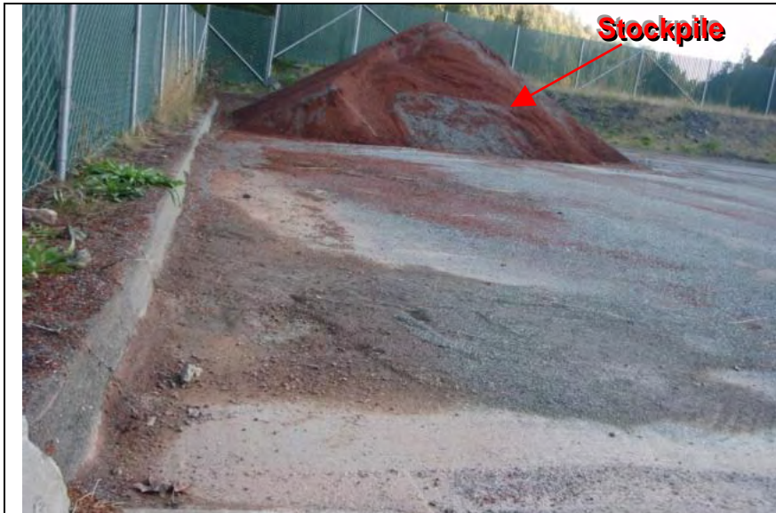
Photograph 1 – Stockpile without BMPs for coverage or containment
