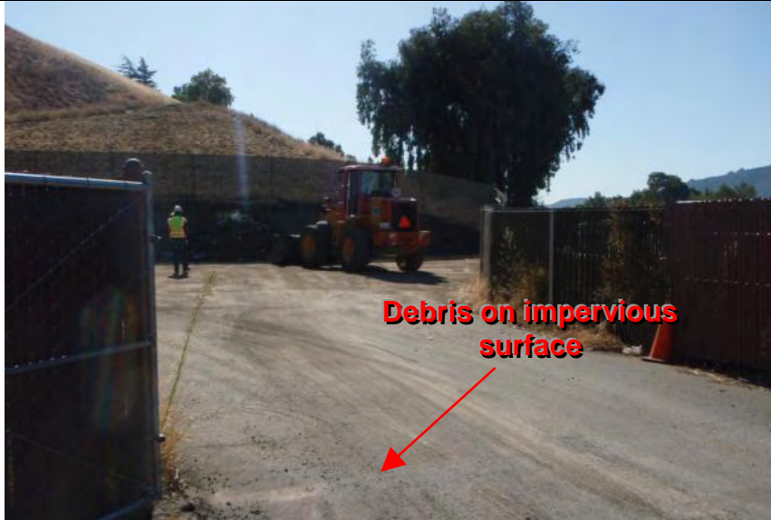
Photograph 1 – Entrance to temporary storage site. (Note: Impervious roadway entrance and tracking of debris)
