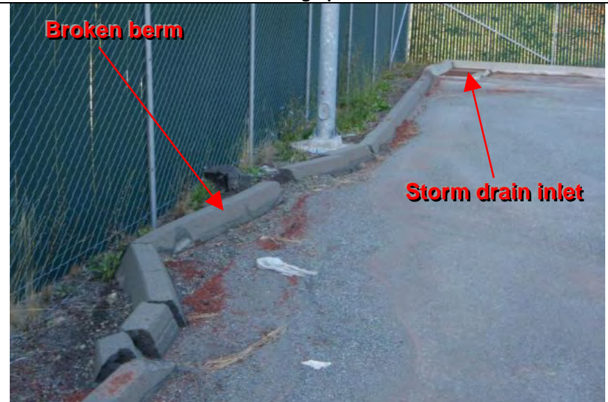
Photograph 4 – Broken berm along northern perimeter of facility (Note: Accumulation of roadway abrasives adjacent to berm)
