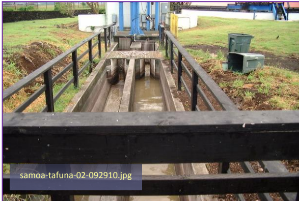
Photo #1: Tafuna STP – Headworks Taken By: Greg V. Arthur Date: 09/29/10
