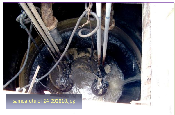
Photo #28: Airport Lift Station (Tafuna service area) Taken By: Greg V. Arthur Date: 09/28/10
