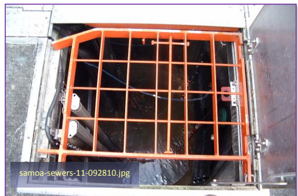
Photo #18: Fatumafuti Lift Station (To Utulei) Taken By: Greg V. Arthur Date: 09/28/10
