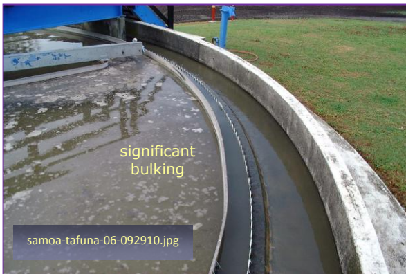
Photo #3: Tafuna STP – Clarigester No.2 Taken By: Greg V. Arthur Date: 09/29/10
