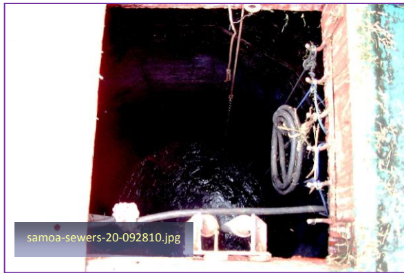
Photo #25: Papa Stream Lift Station (To Tafuna) Taken By: Greg V. Arthur Date: 09/28/10
