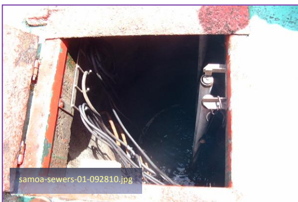
Photo #11: Atu'u Lift Station (Utulei service area) Taken By: Greg V. Arthur Date: 09/28/10
