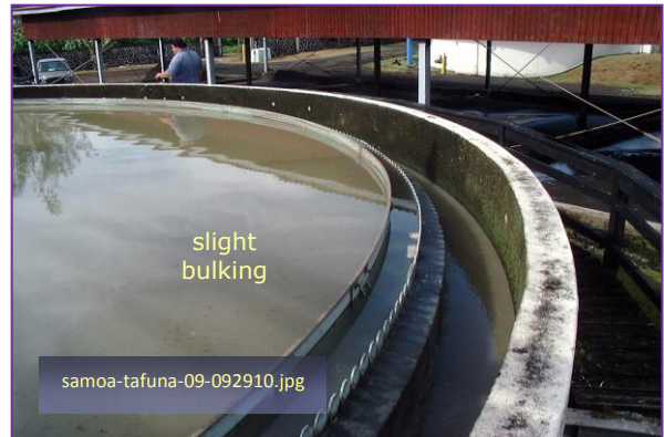
Photo #2: Tafuna STP – Clarigester No.1 Taken By: Greg V. Arthur Date: 09/29/10
