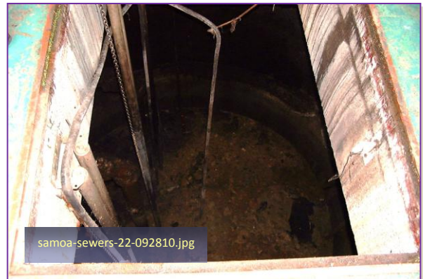
Photo #26: Vaitele Main Lift Station (To Tafuna) Taken By: Greg V. Arthur Date: 09/28/10
