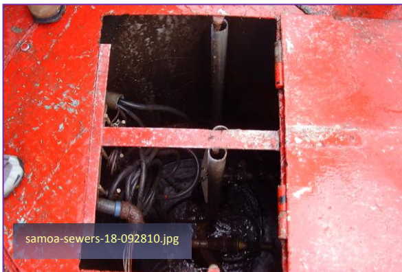
Photo #23: Andy Lift Station (Tafuna service area) Taken By: Greg V. Arthur Date: 09/28/10
