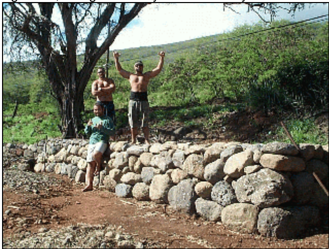
Figure 55, Kalaniua Ritte, Joshua Kalua and Guy Naehu Show off the Rock Wall they Constructed for the Native Plan Garden at Keawanui.
