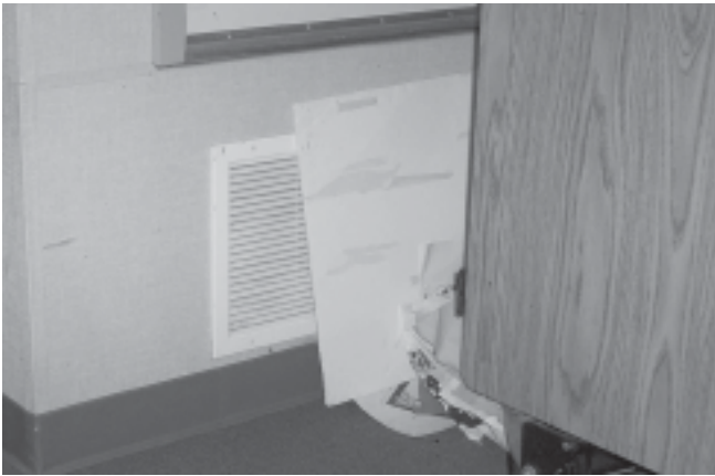
US EPA funded indoor air quality assessments at seven schools in the Ravenswood City School District. Blocked vents were one of several problems detected that can contribute to poor air quality and can worsen asthma.
