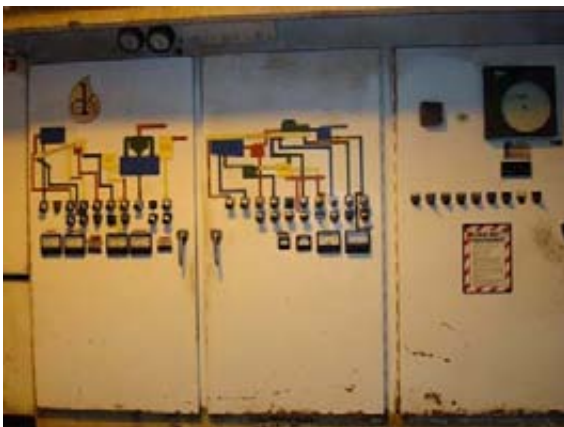
Control Panel for Pretreatment Processes
