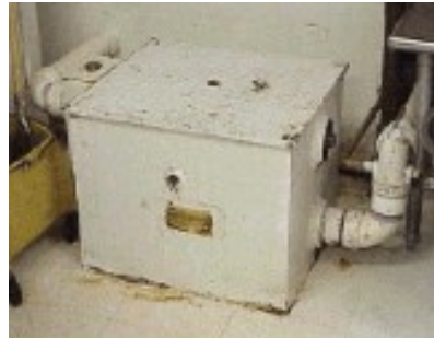
Figure 2. Picture of an interior grease trap. Small grease traps are sufficient for low volume producers and may require as frequent as weekly maintenance.
