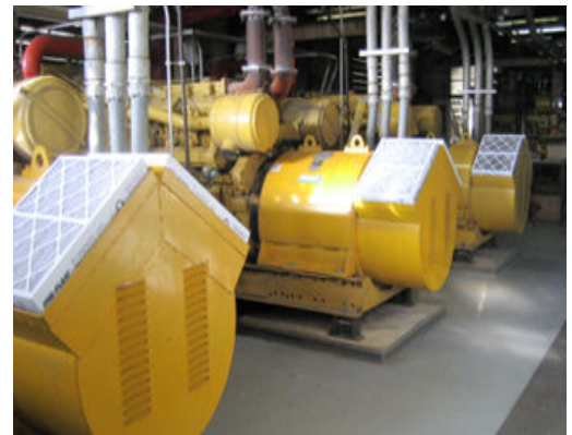
Figure 9. An example cogeneration system that resembles the one found at the City of Santa Cruz Waste Water Treatment Plant.
