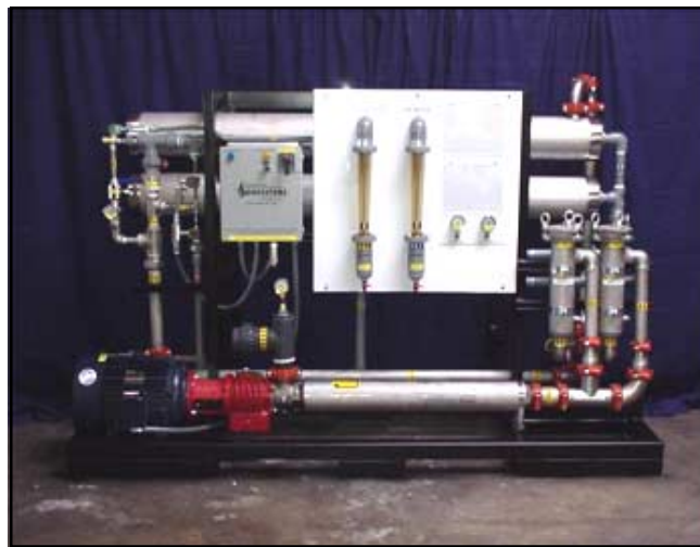
Figure 3. Perfection Plating's RO System
