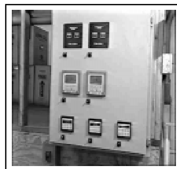
Figure 6. Analyzer Panel at the Artistic Facility
